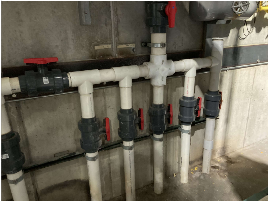
Title: Kwik Trip Bakery Expansion/0632560495/20220926/right bank of VMS manifold piping - all valves open
