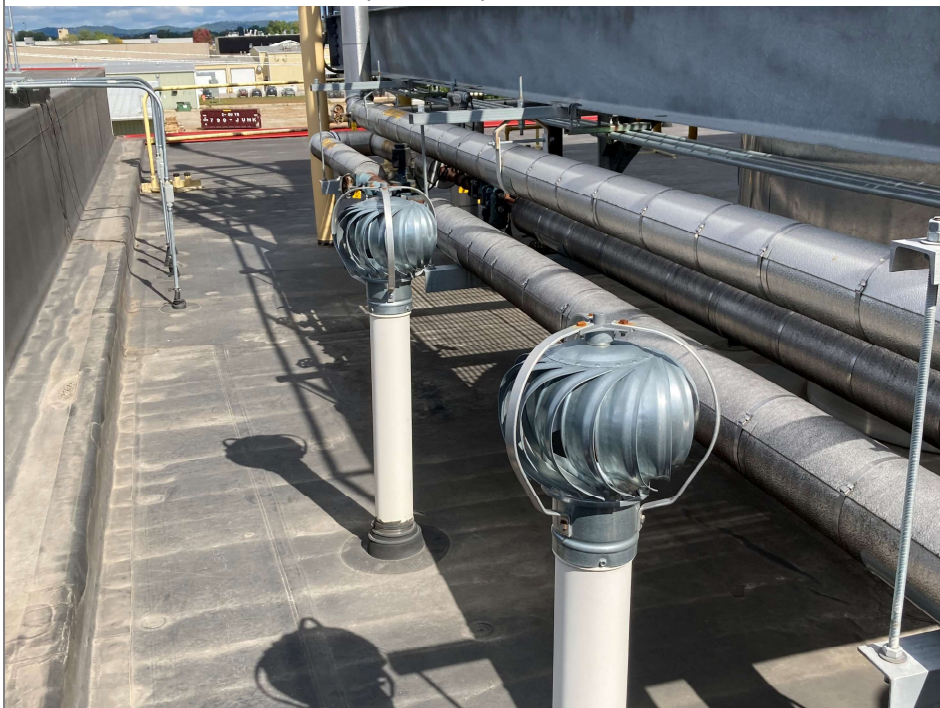
Title: Kwik Trip Bakery Expansion/0632560495/20220926/VMS exhaust with wind turbines functioning properly
