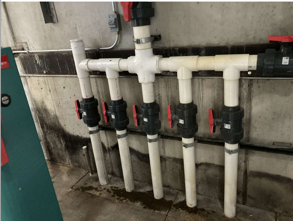
Title: Kwik Trip Bakery Expansion/0632560495/20220926/left bank of VMS manifold piping - all valves open
