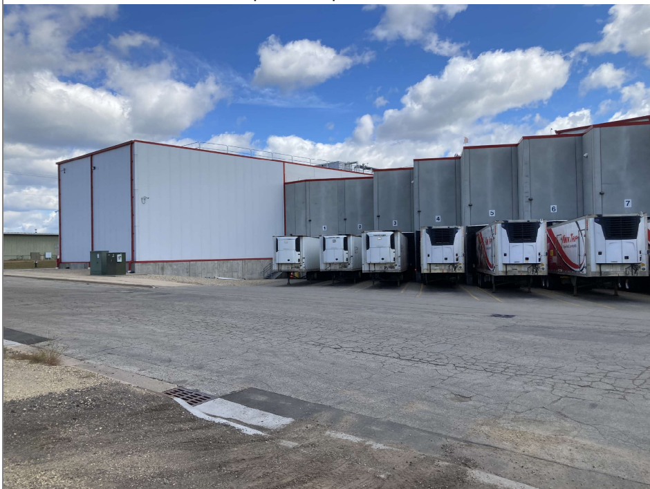
Title: Kwik Trip Bakery Expansion/0632560495/20220926/Loading dock area - west end of bakery expansion
