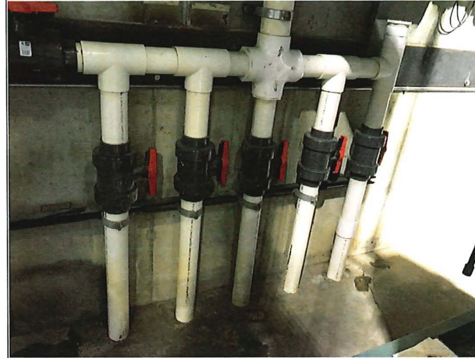
Title: VMS manifold piping - all valves open
