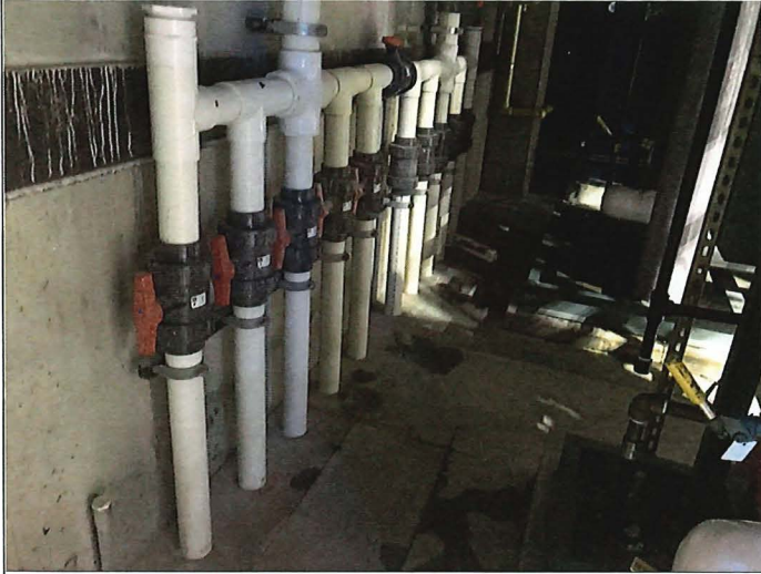
Title: VMS manifold piping - all valves open
