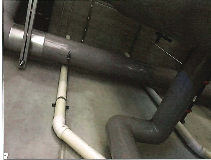
Title: VMS piping to roof
