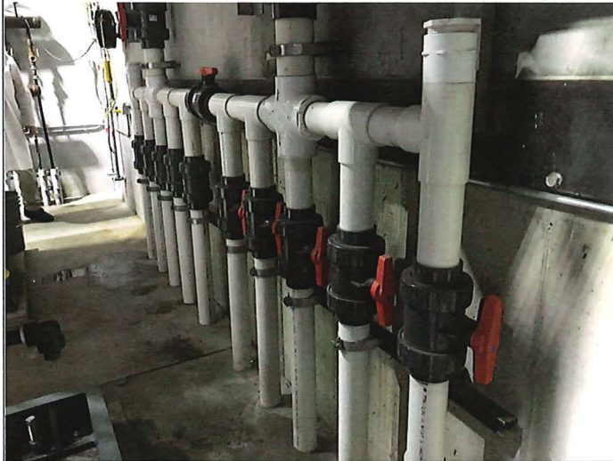
Title: VMS manifold piping - all valves open
