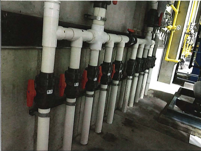
Title: VMS manifold piping - all valves open
