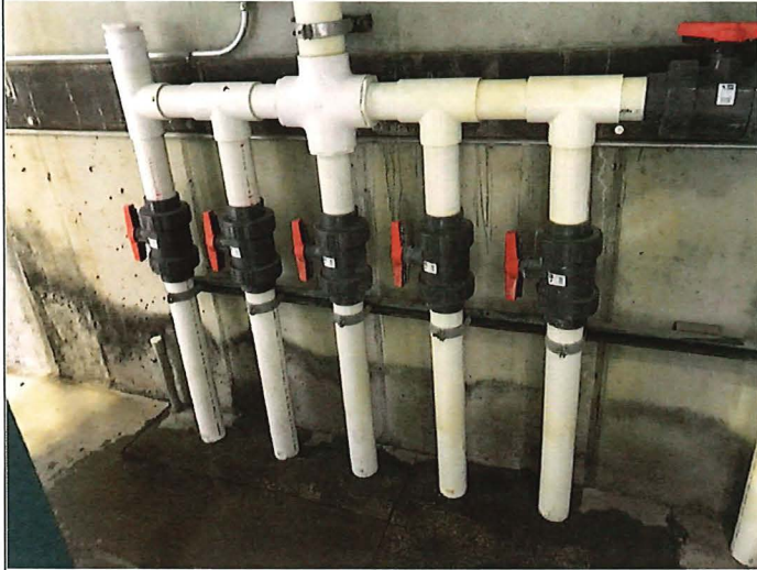
Title: VMS manifold piping - all valves open
