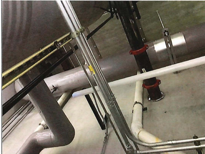
Title: VMS exhaust piping to roof
