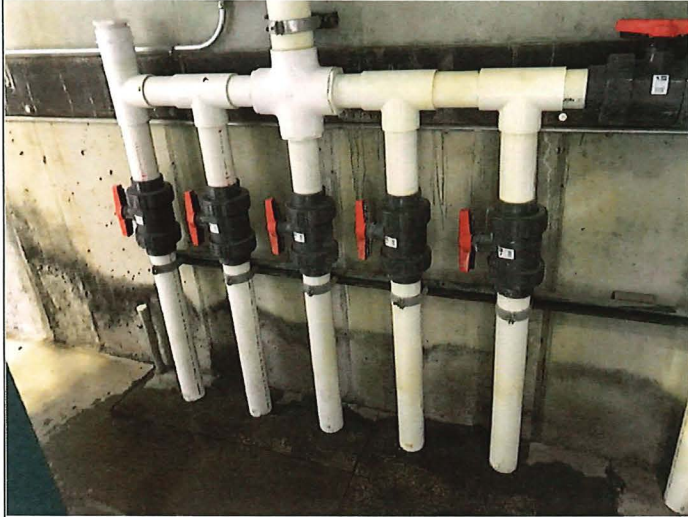
Title: VMS manifold piping - all valves open
