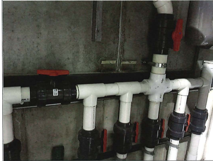
Title: VMS manifold piping - all valves open
