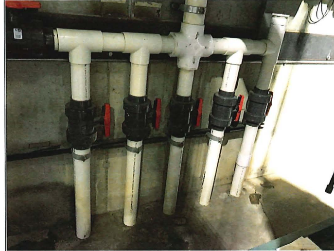
Title: VMS manifold piping - all valves open
