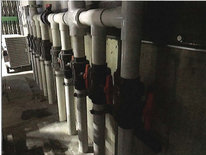
Title: VMS manifold piping - all valves open
