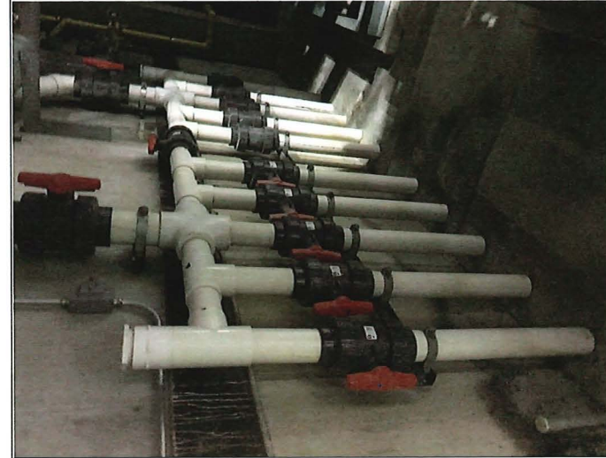
Title: VMS manifold piping - all valves open
