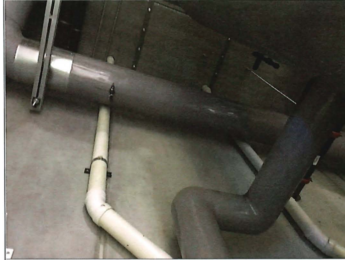
Title: VMS piping to roof
