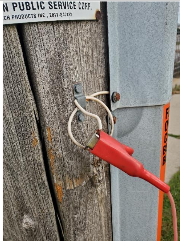
Transmitter Connection Closeup – Fiber Optic Connection
