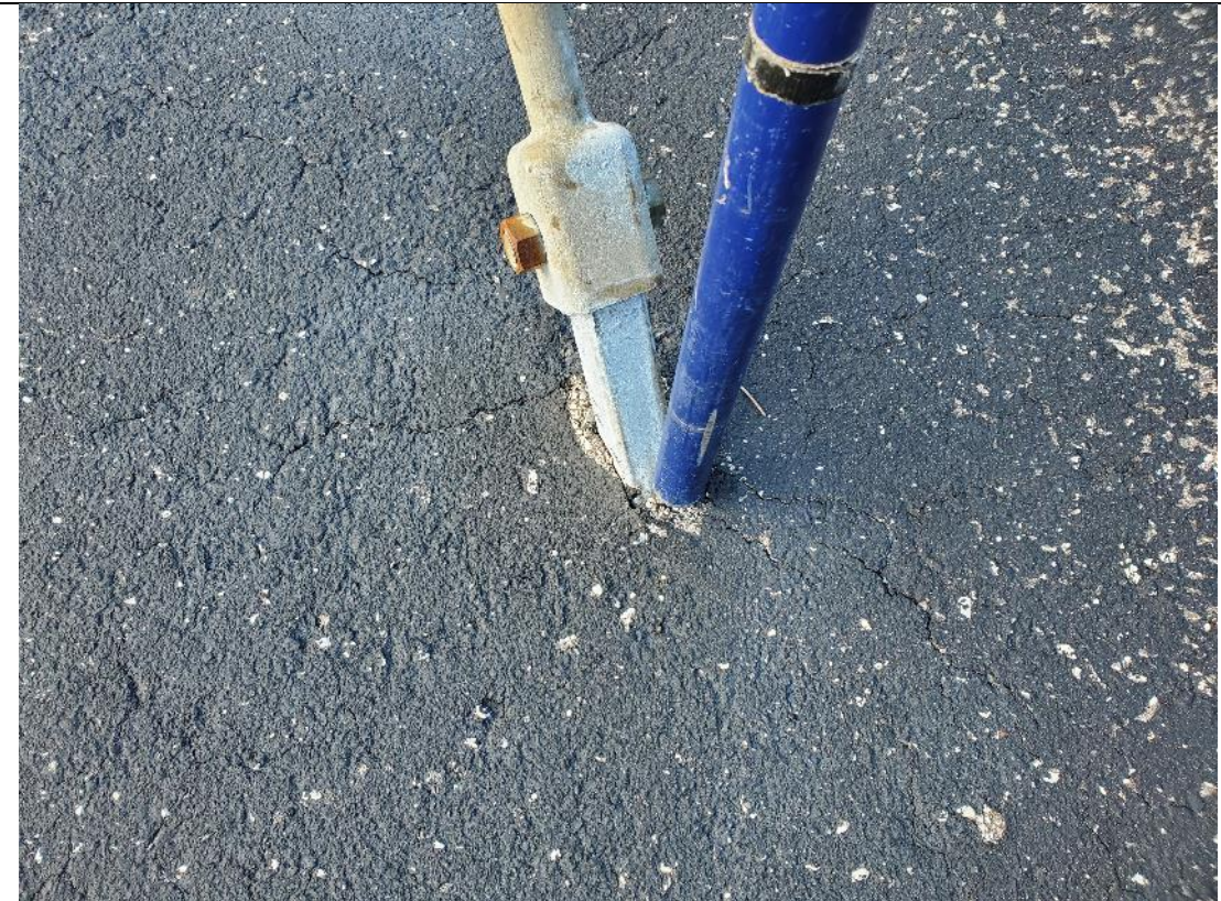
Control Point "CO1" Closeup
