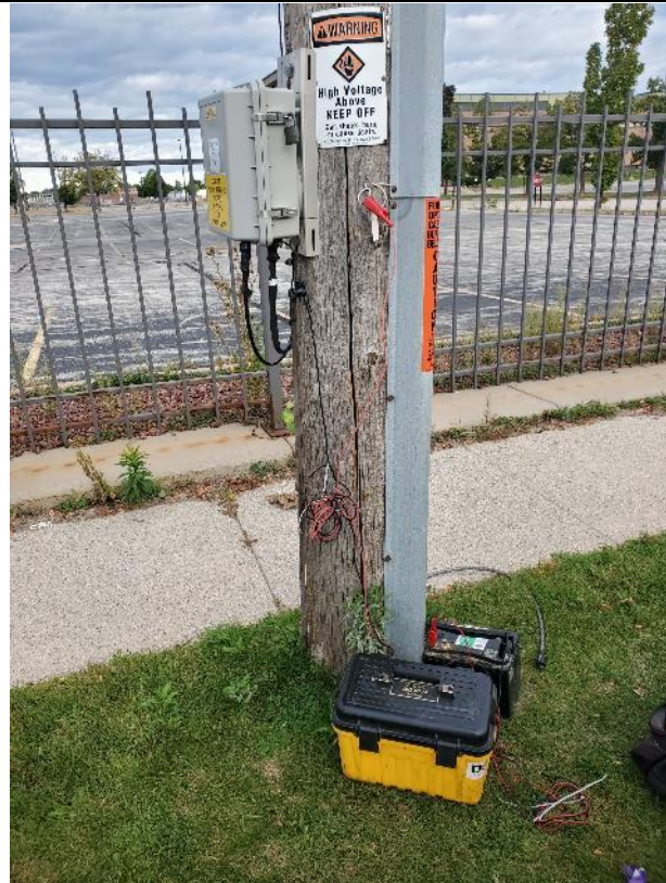
Transmitter Connection Site Overview
