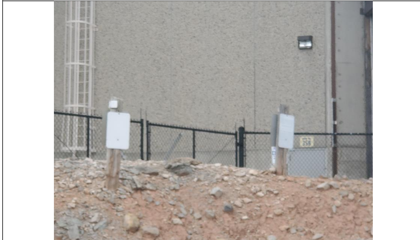
Eastern Shore signage for buried cable
