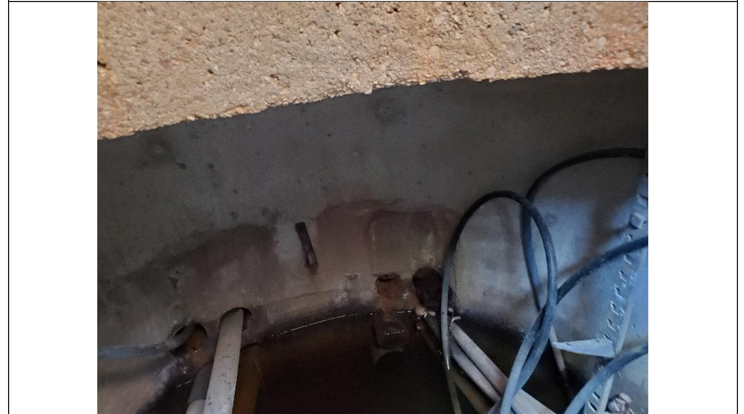
Cables in Western shore vault, possibly heading to signs on Eastern shore
