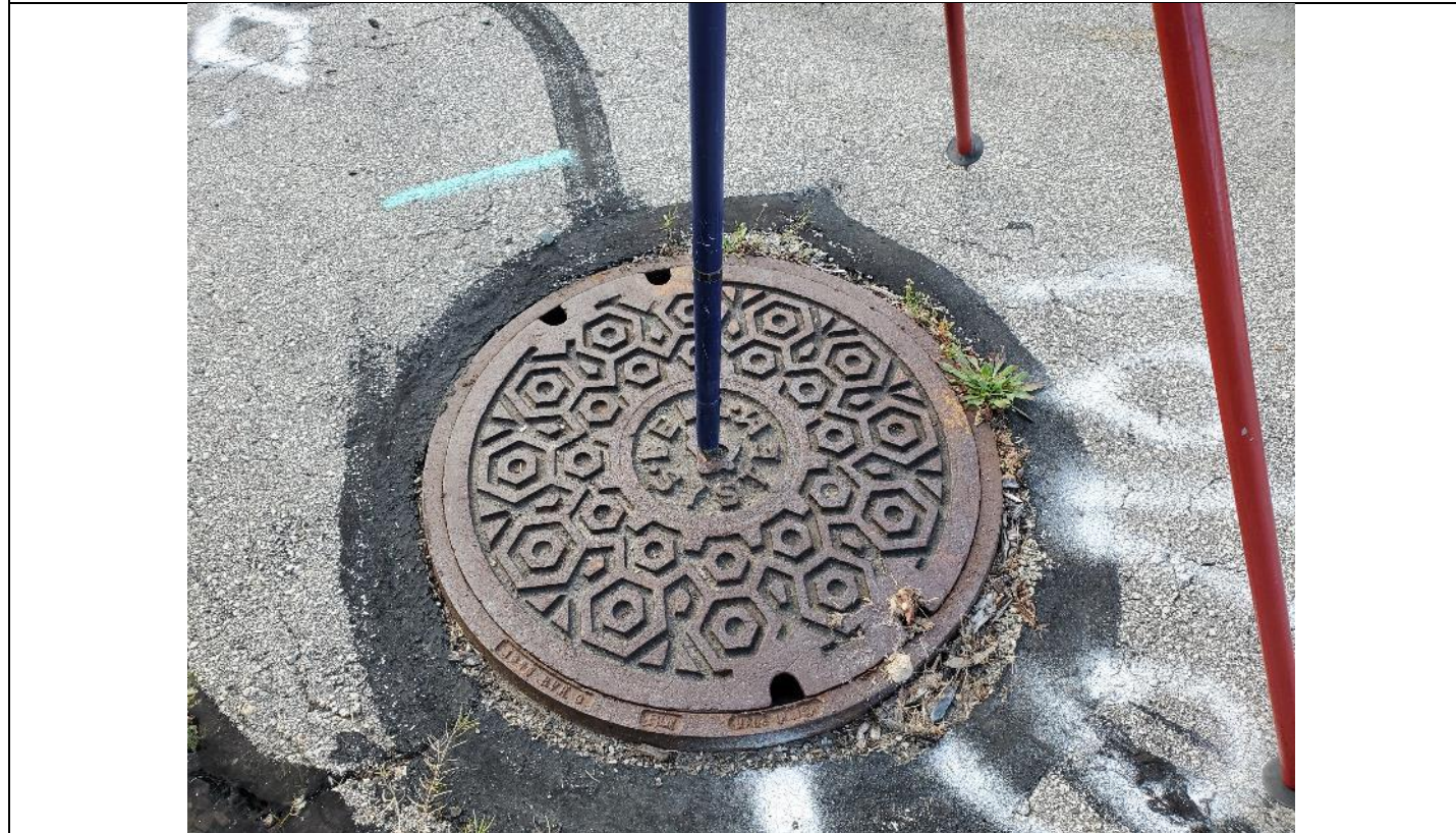
Control Point "CO2" Closeup
