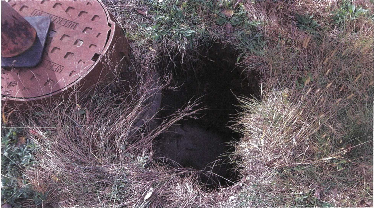
Erosion by EW-5
