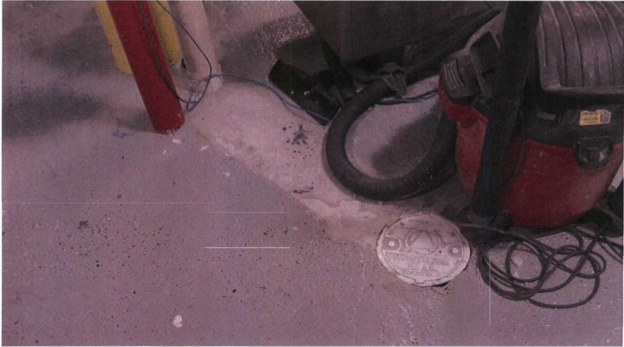
Building 105 SVE System Intake
