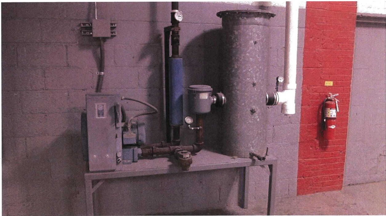
Building 105 SVE System
