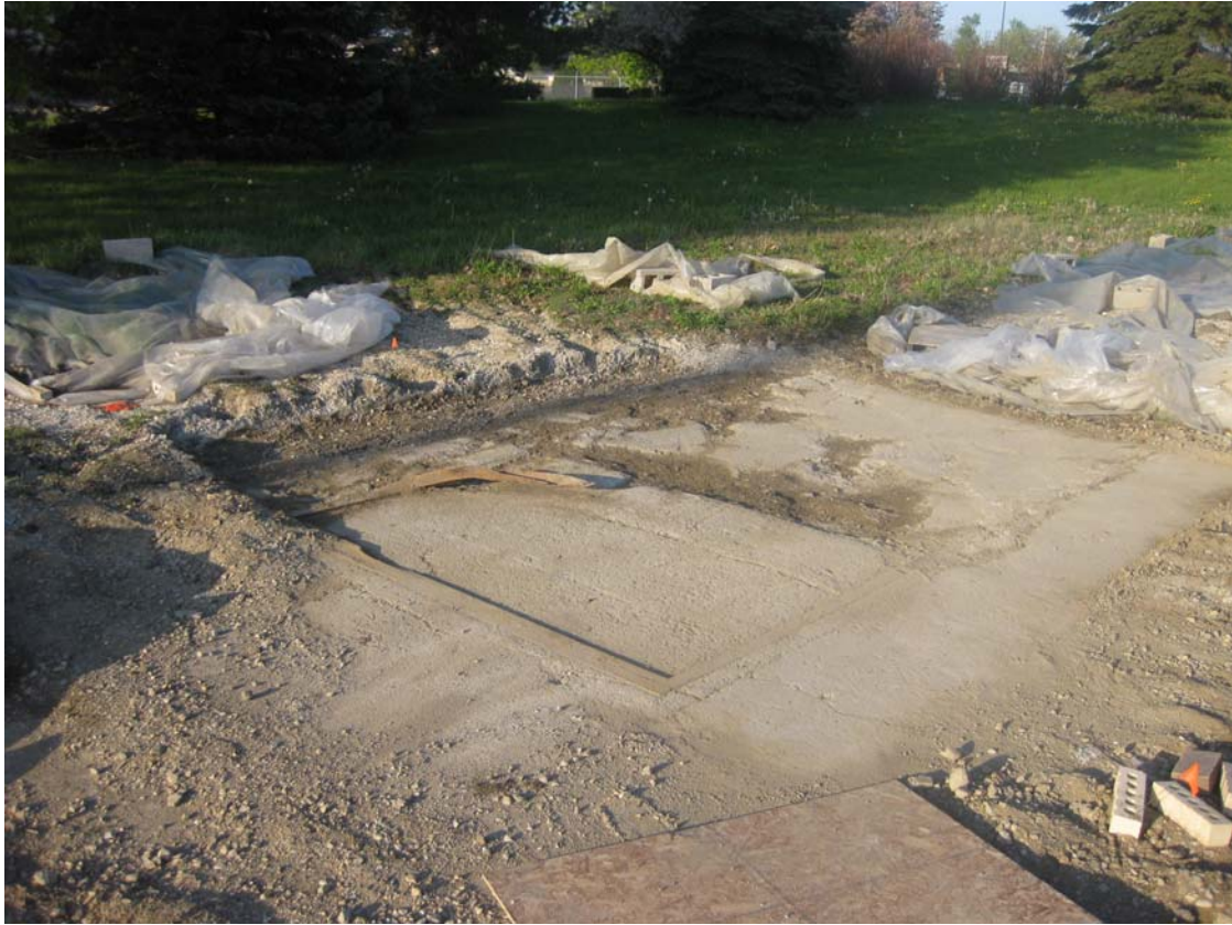
Photo 7 - Soil Pile Area C-10 (plus a half node) Looking Northeast (after final sweeping)
