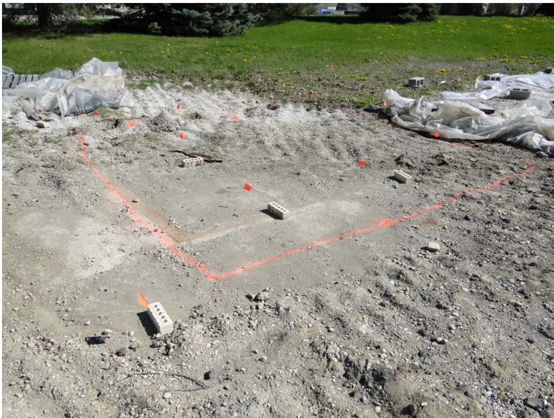
Photo 6 - Soil Pile Area C-10 (plus a half node 0.75 M) Looking North (prior to final sweeping)
