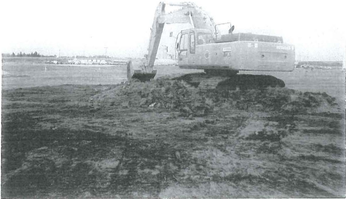
Photograph shows the removal of sod from the surface of an area to be excavated.
