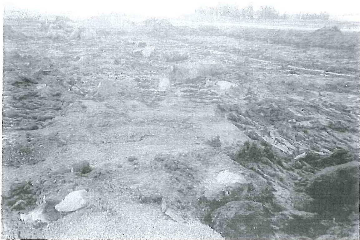
Photograph shows an area of gravel fill and several concrete foundations. Such material and items were stockpiled to the side of the excavation and were not transported to the landfill.
