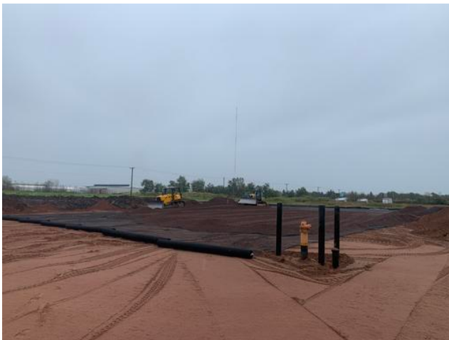
Hydrant Bollards & GeoGrid on Van Lot
