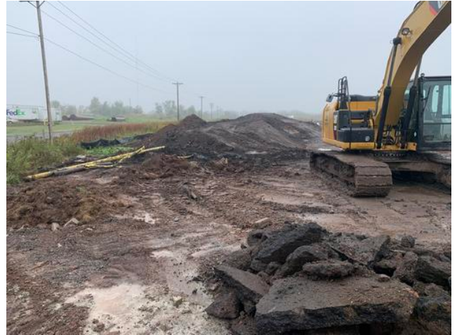
Pond berm & debris
