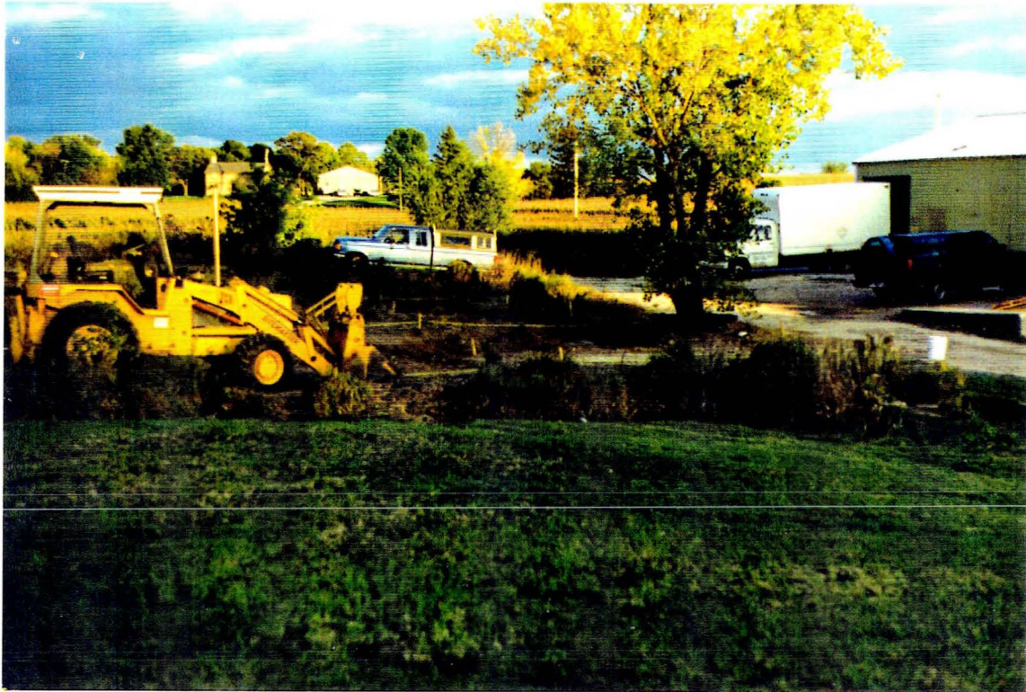
PHOTOGRAPH #1: LOOKING SOUTHEAST AT EXCAVATION IN WAX STORAGE AREA ORIGINAL TRAILER AREA EXCAVATION IS BETWEEN TREE BOX AND BLUE TRUCK
