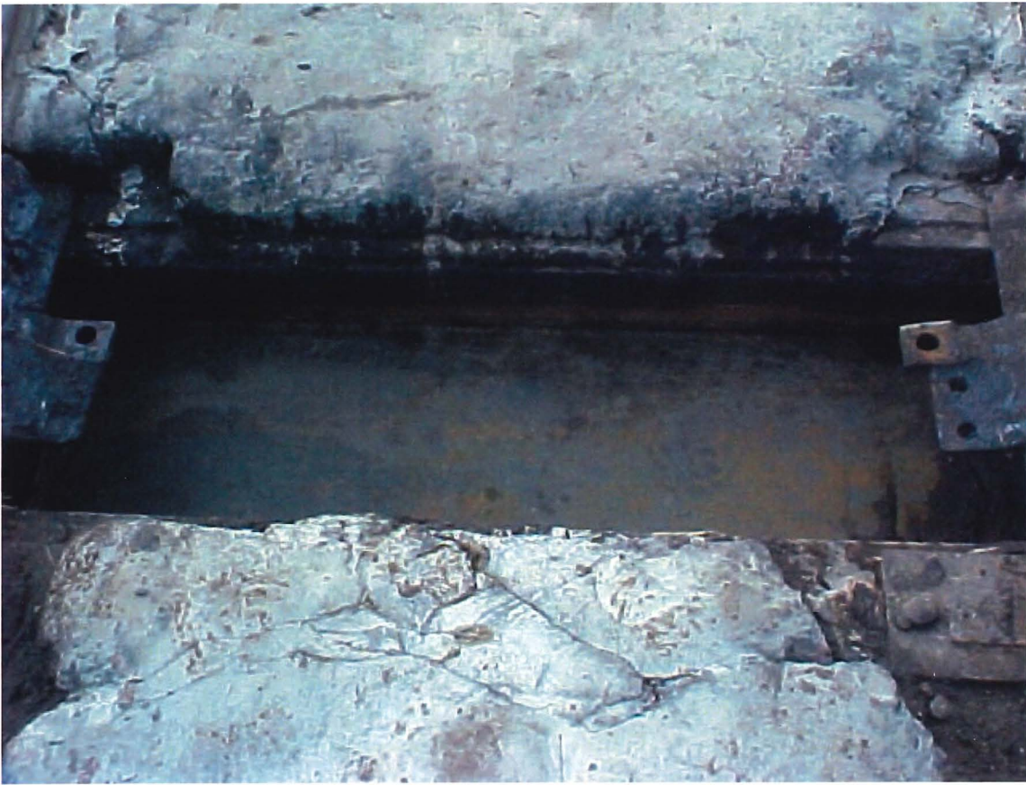
One of the catch basins
