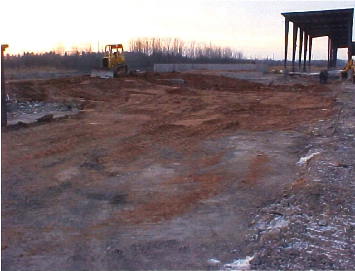
Tank farm and treating building area filled with clean sand prior to concrete cap.
