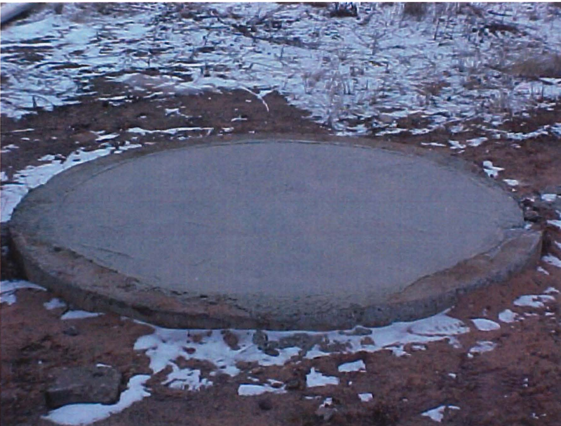
Sumps along drip pad filled with sand and topped with concrete cap to prevent water collection.
