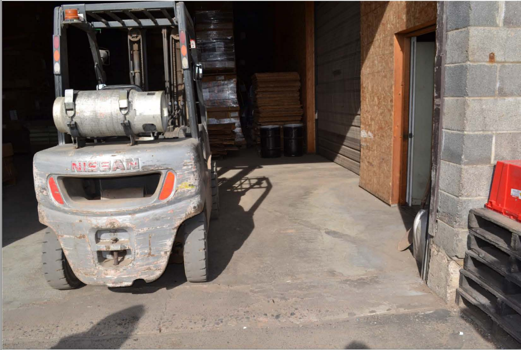
Title: Doberstein looking west into the building at the floor sealant that needs repairs
