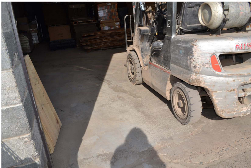
Title: Doberstein looking west into the building at the floor sealant that needs repairs
