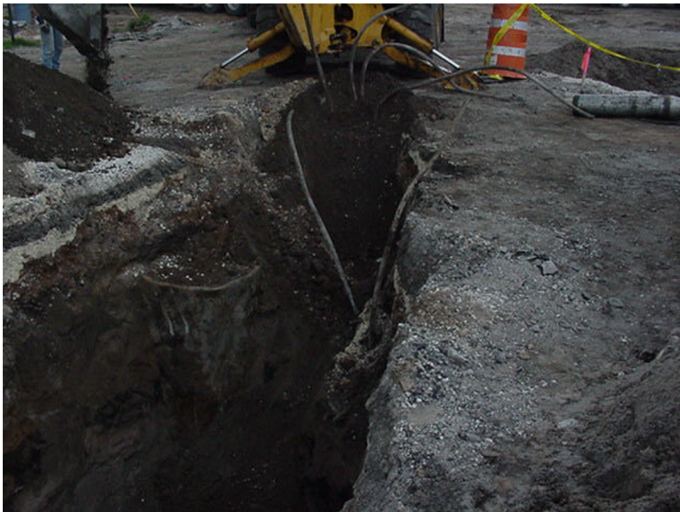
Photograph 4: UST #3 and associated piping.
