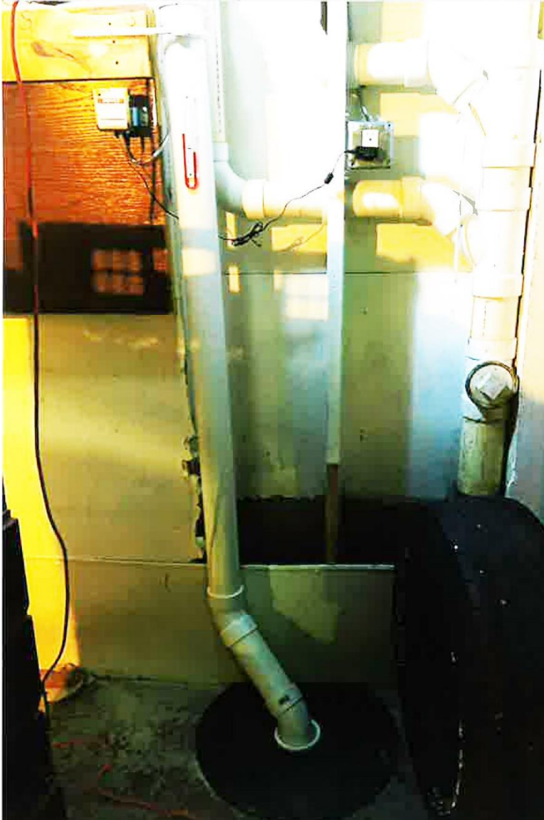
Photo 3: Seal and piping at Pickup Point 1.
