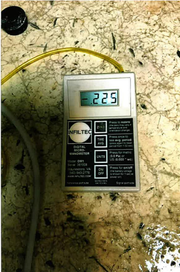
Photo 13: Sub-slab vacuum at VOP-2 following system startup.
