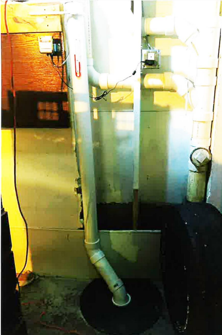
Photo 3: Seal and piping at Pickup Point 1.
