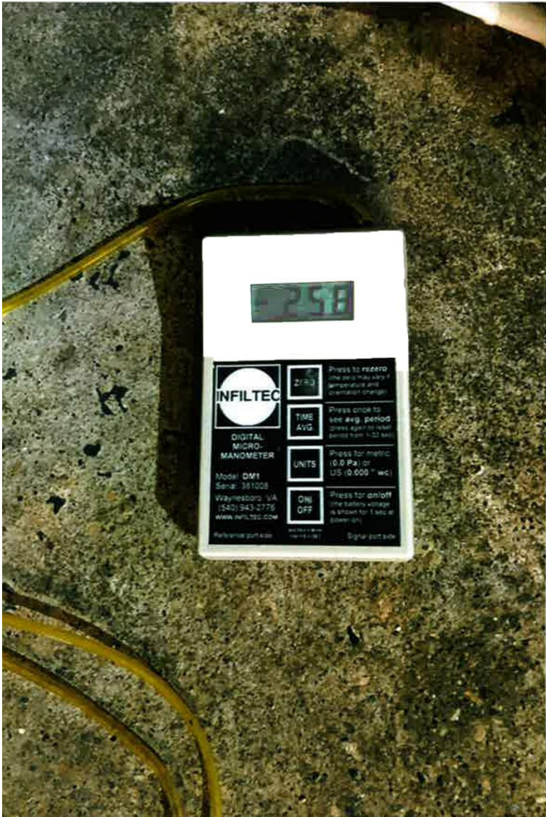
Photo 12: Sub-slab vacuum in inches of water at VOP-1 following system startup.
