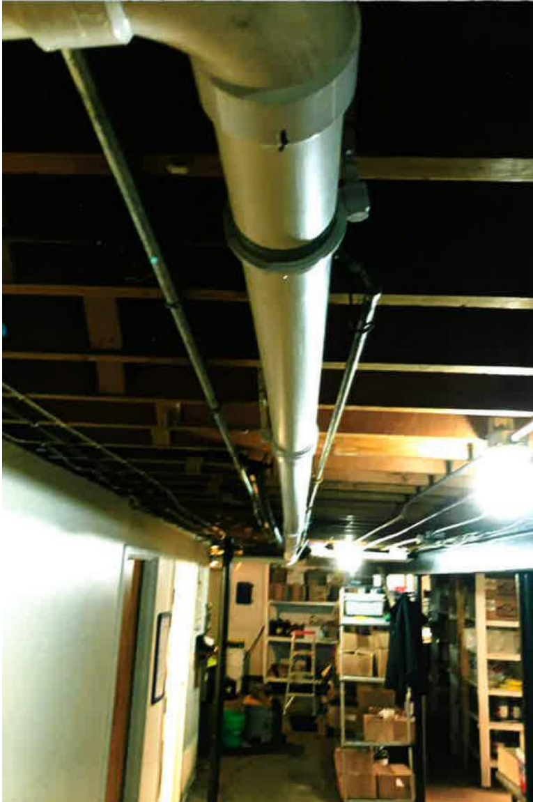
Photo 6: Piping run from Pickup Point 2.
