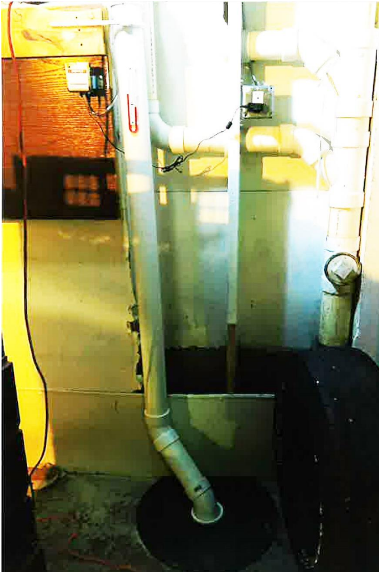
Photo 3: Seal and piping at Pickup Point 1.
