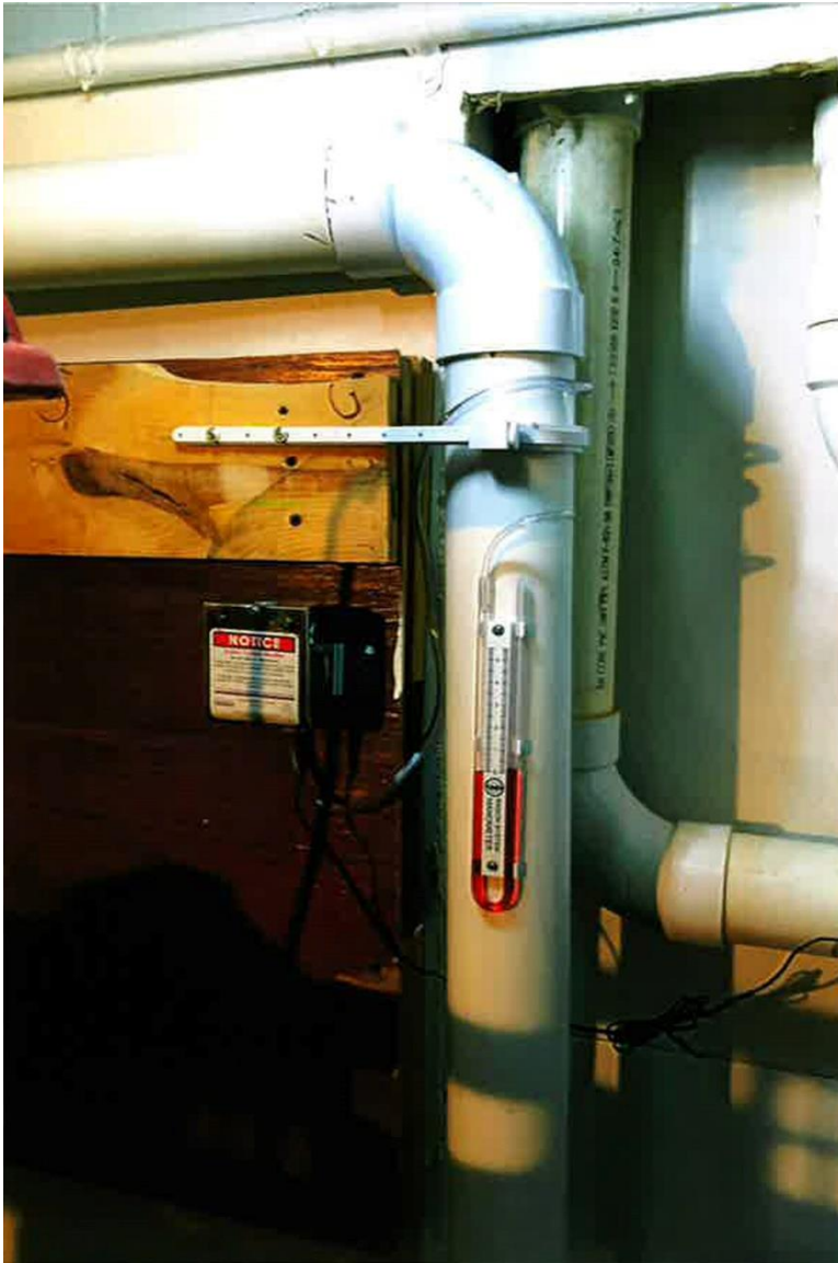
Photo 4: Manometer and system alarm at Pickup Point 1.
