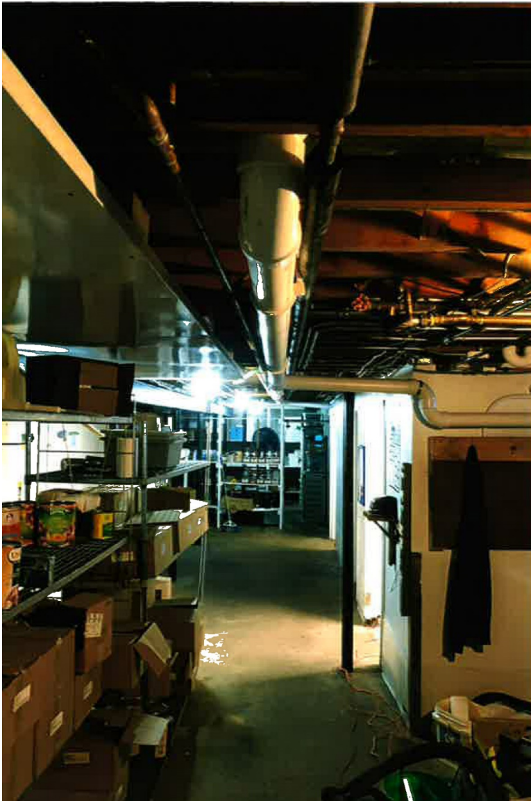
Photo 7: Piping run from Pickup Point 1.
