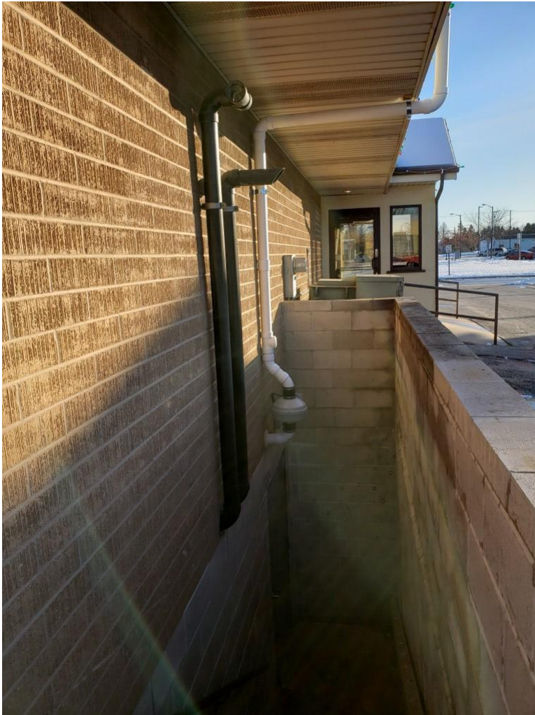
Photo 15: Vapor mitigation system fan and exhaust.
