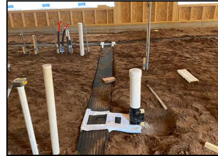
Riser and Gas Mat
