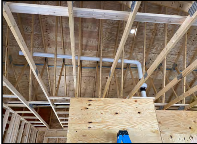
Riser capped and blower above drop ceiling
