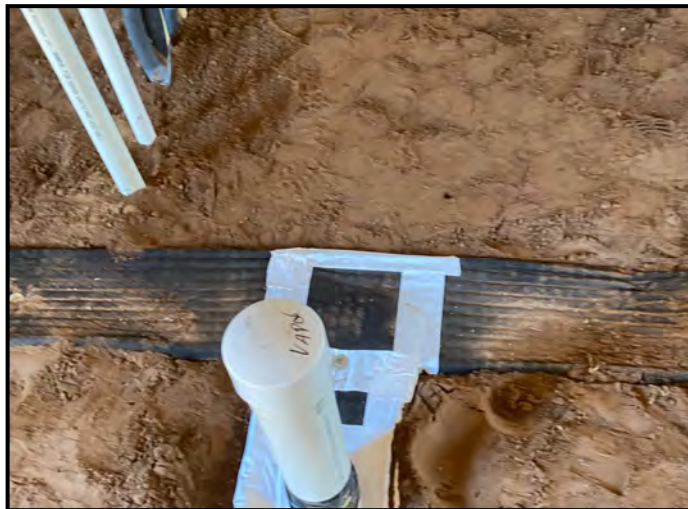
Riser connection to Gas Mat
