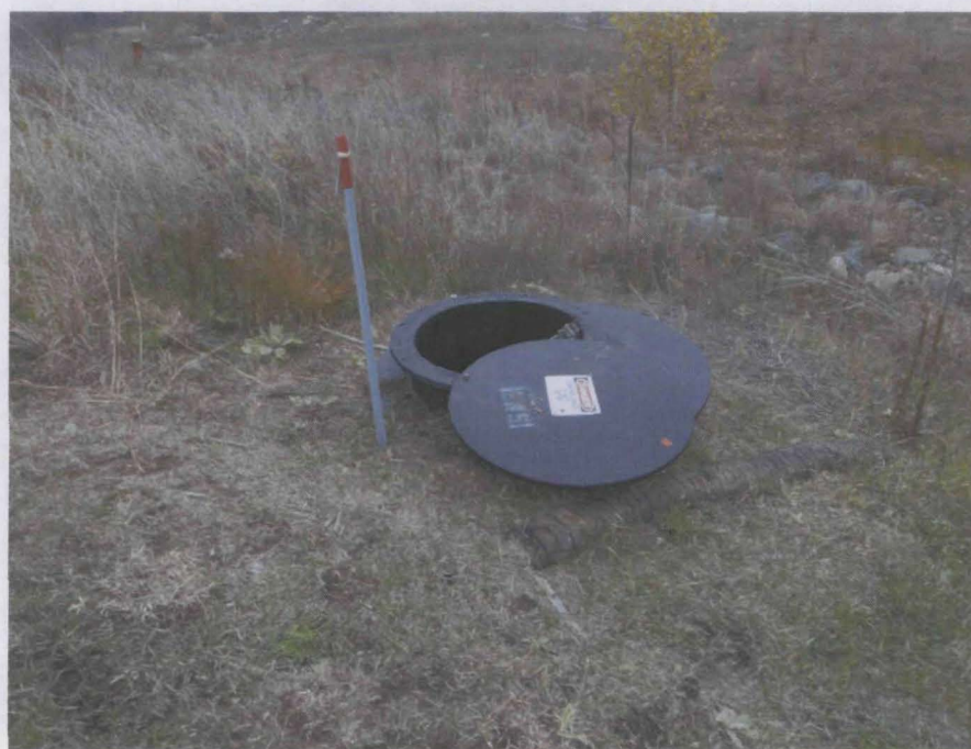
LNAPL Extraction Well
