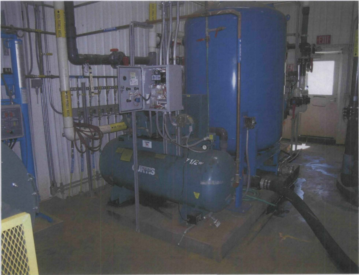
Compressor and Air Dryer
