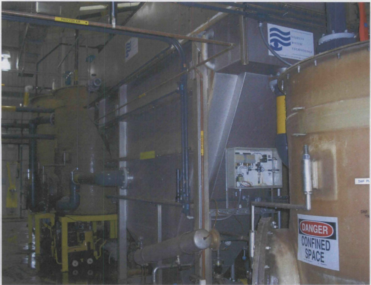
From Right, Equalization Tank, Dissolved Air Flootation Unit, Coagulant Reaction Tank, Flocculant Reaction Tank
