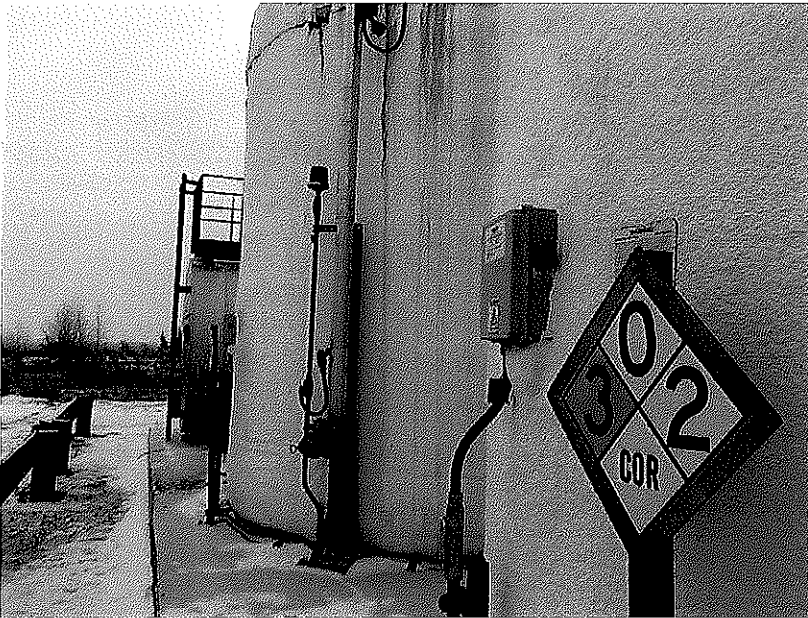
Picture 23: Outdoor Storage Tanks
