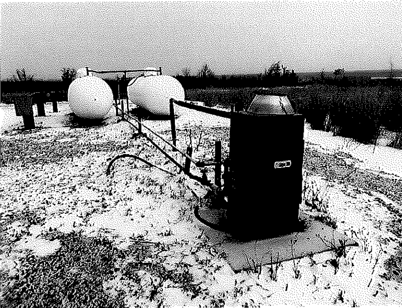
Picture 22: Propane tanks and furnace
