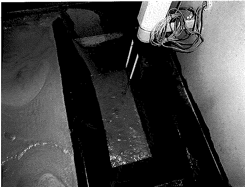
Picture 6: DAF sludge blanket/probes
