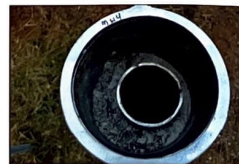
SEAM-CONFINED MONITORING WELL
