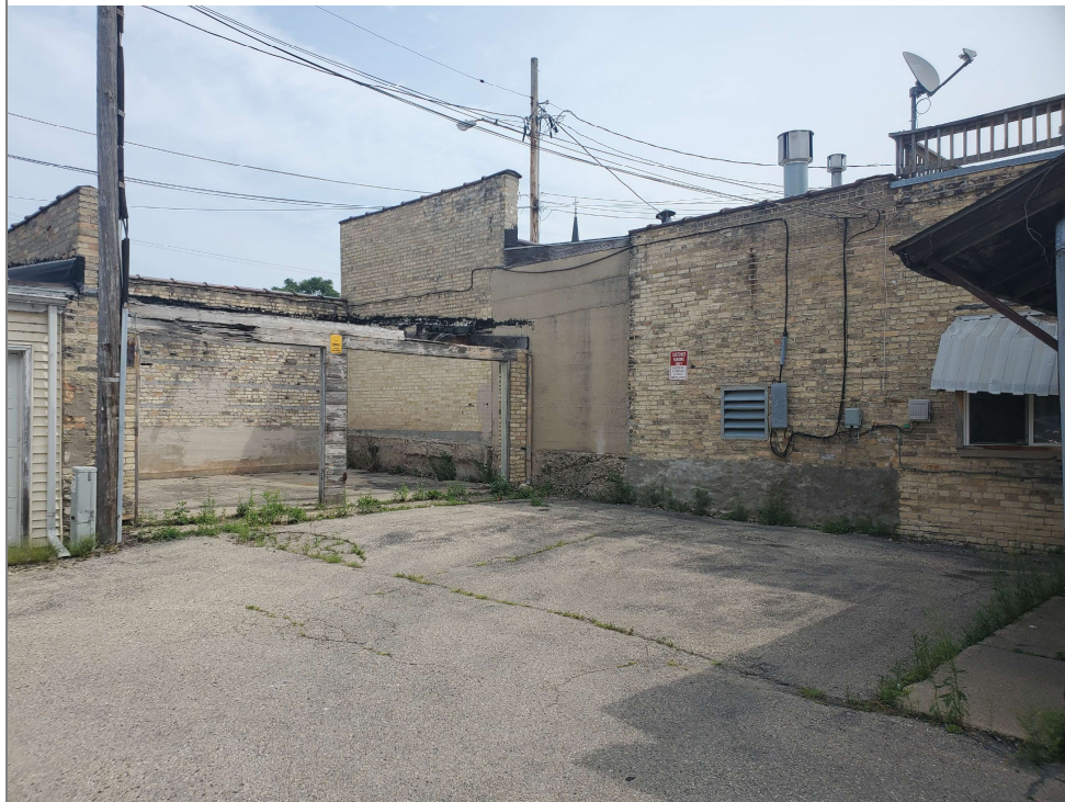
Title: looking northeast at building in the area of the residual soil contamination.
