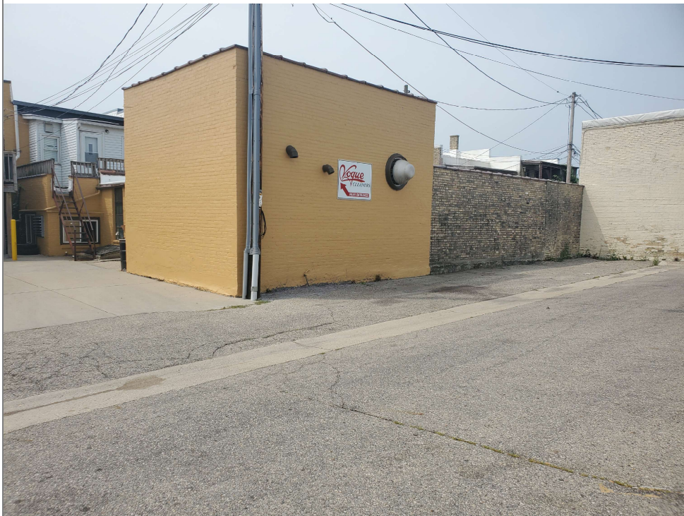
Title: looking southwest at the building in the area of residual soil contamination
