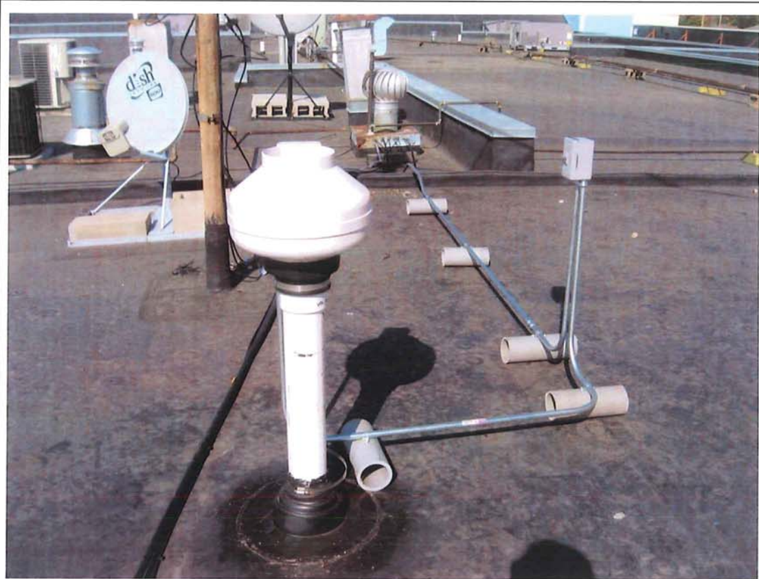
Photograph #: 7 Date: 10/5/2012 Direction: System #1 Subject: Fan mounted on roof with on/off switch
