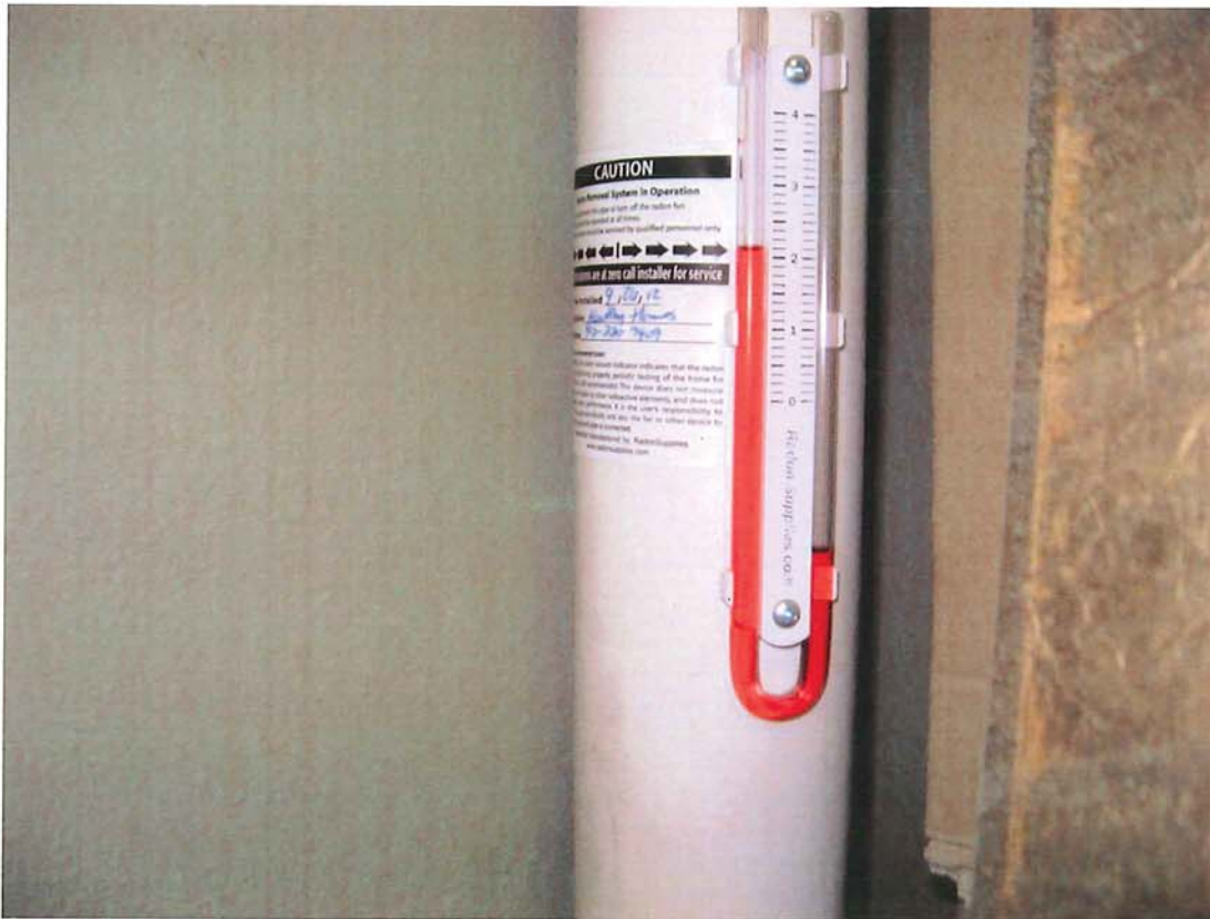
Photograph #: 14 Date: 10/26/2012 Direction: System #3 Subject: U-tube monometer
