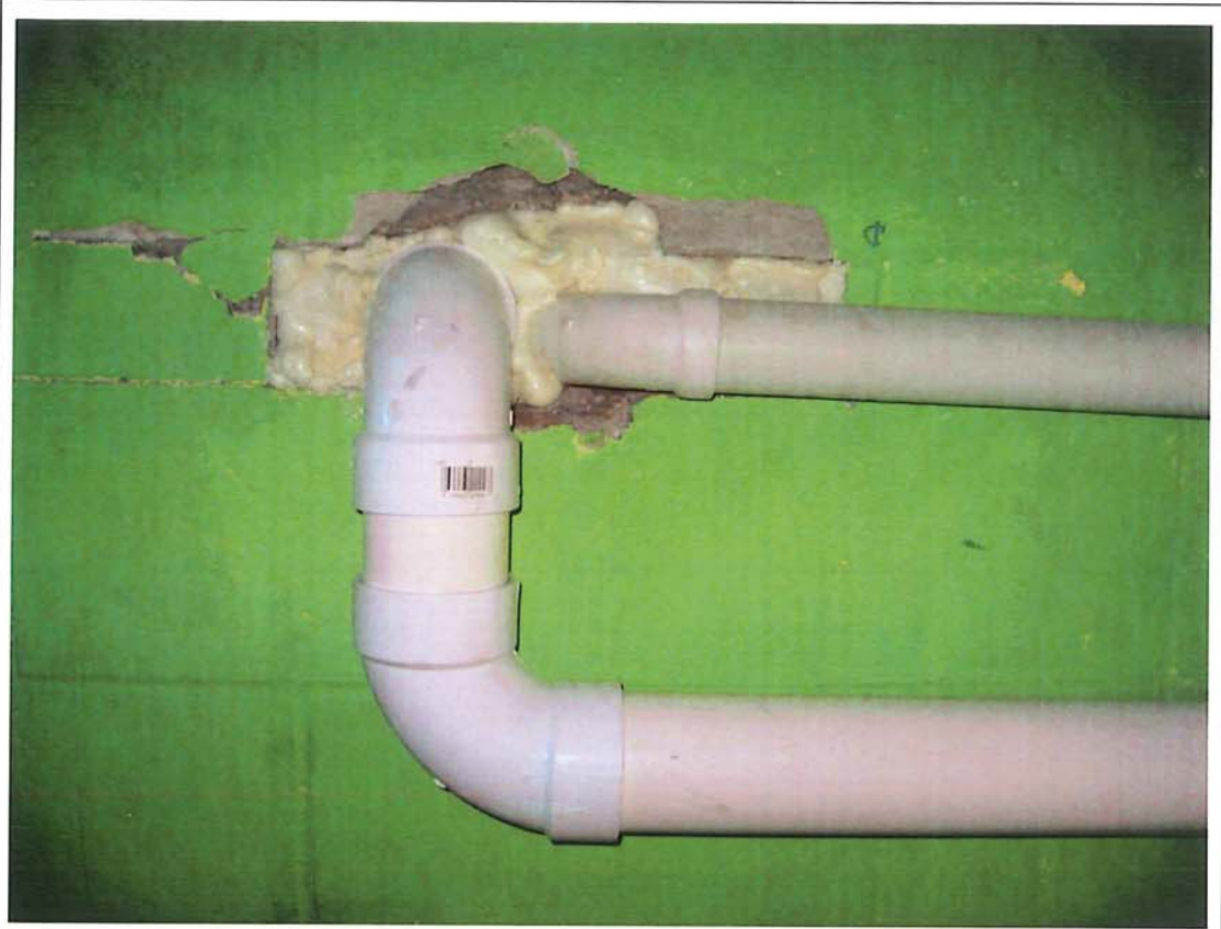
Photograph #: 5 Date: 9/26/2012 Direction: System #2 Subject: Block wall suction point in stairwell (small pvc pipe is septic)
