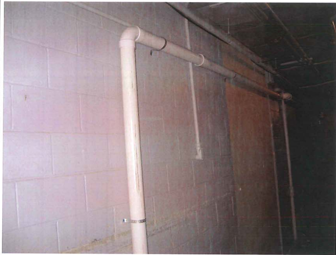
Photograph #: 3 Date: 5/24/2011 Direction: 9/25/2012 Subject: Piping manifolded together
