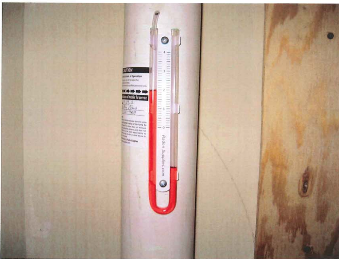
Photograph #: 16 Date: 10/26/2012 Direction: System #5 Subject: U-tube monometer
