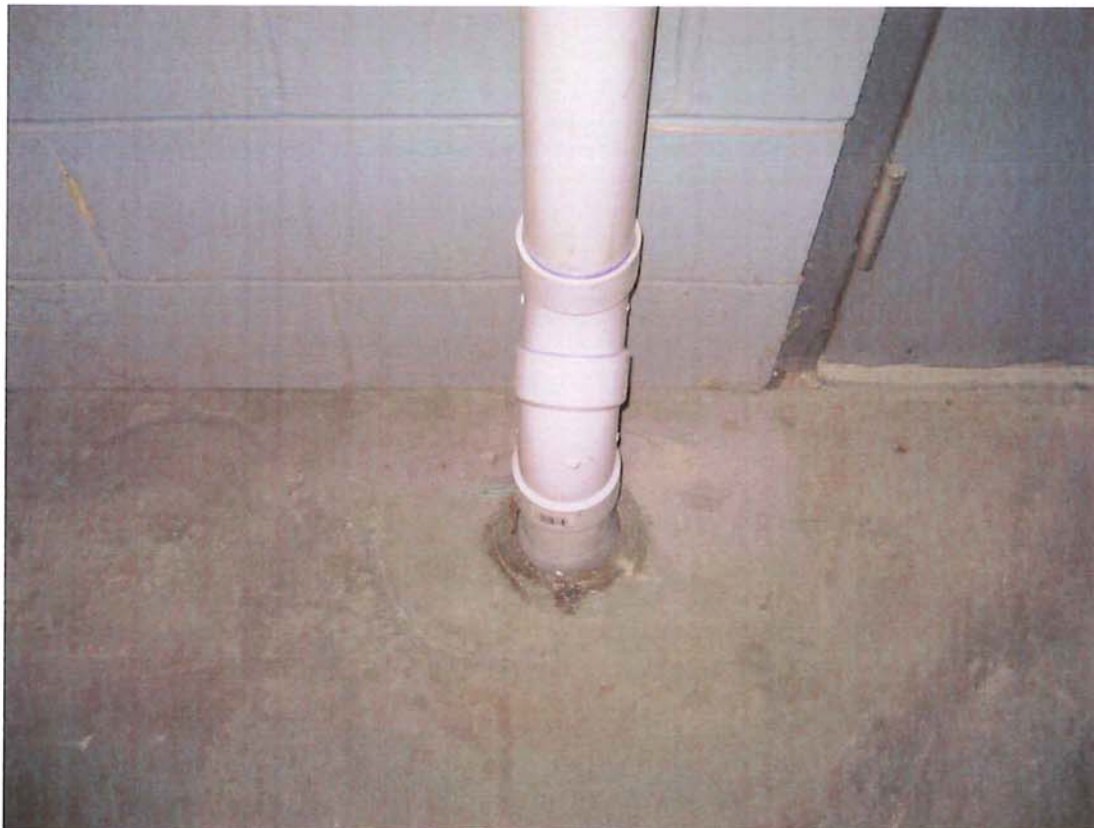
Photograph #: 2 Date: 9/25/2012 Direction: System #1 Subject: Sub-slab depressurization system suction point
