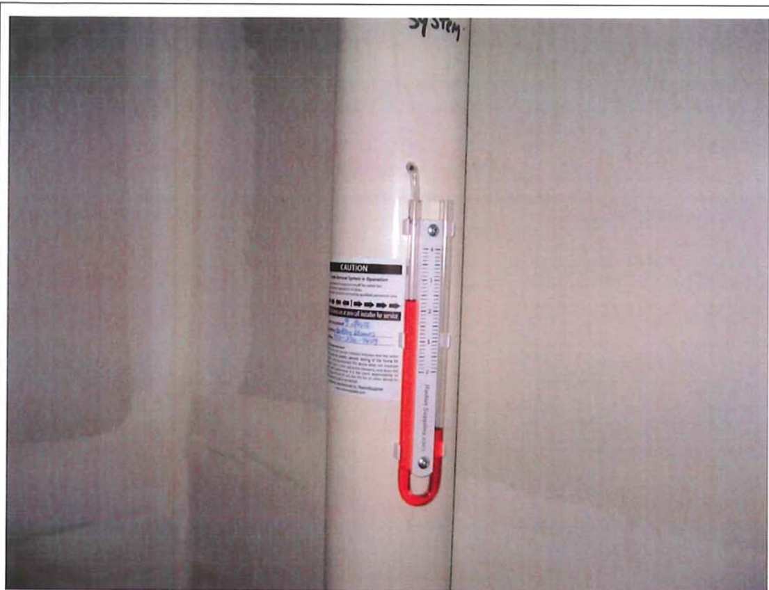
Photograph #: 15 Date: 10/26/2012 Direction: System #4 Subject: U-tube monometer
