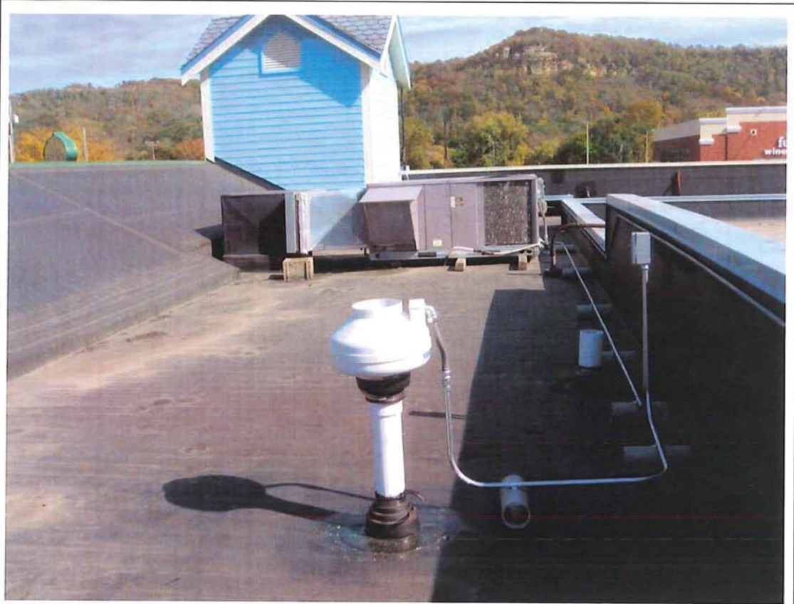
Photograph #: 9 Date: 10/5/2012 Direction: System #3 Subject: Fan mounted on roof with on/off switch
