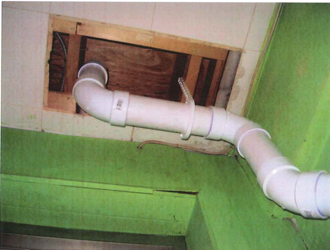
Photograph #: 6 Date: 9/26/2012 Direction: System #2 Subject: Piping routed to roof
