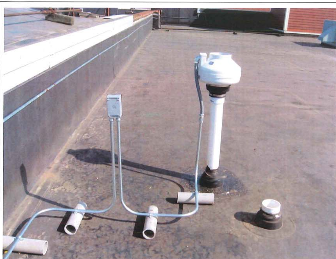
Photograph #: 11 Date: 10/5/2012 Direction: System #5 Subject: Fan mounted on roof with on/off switch
