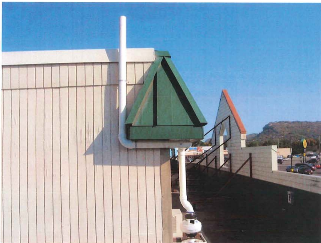
Photograph #: 8 Date: 9/28/2012 Direction: System #2 Subject: Fan mounted on roof with exhaust above eave
