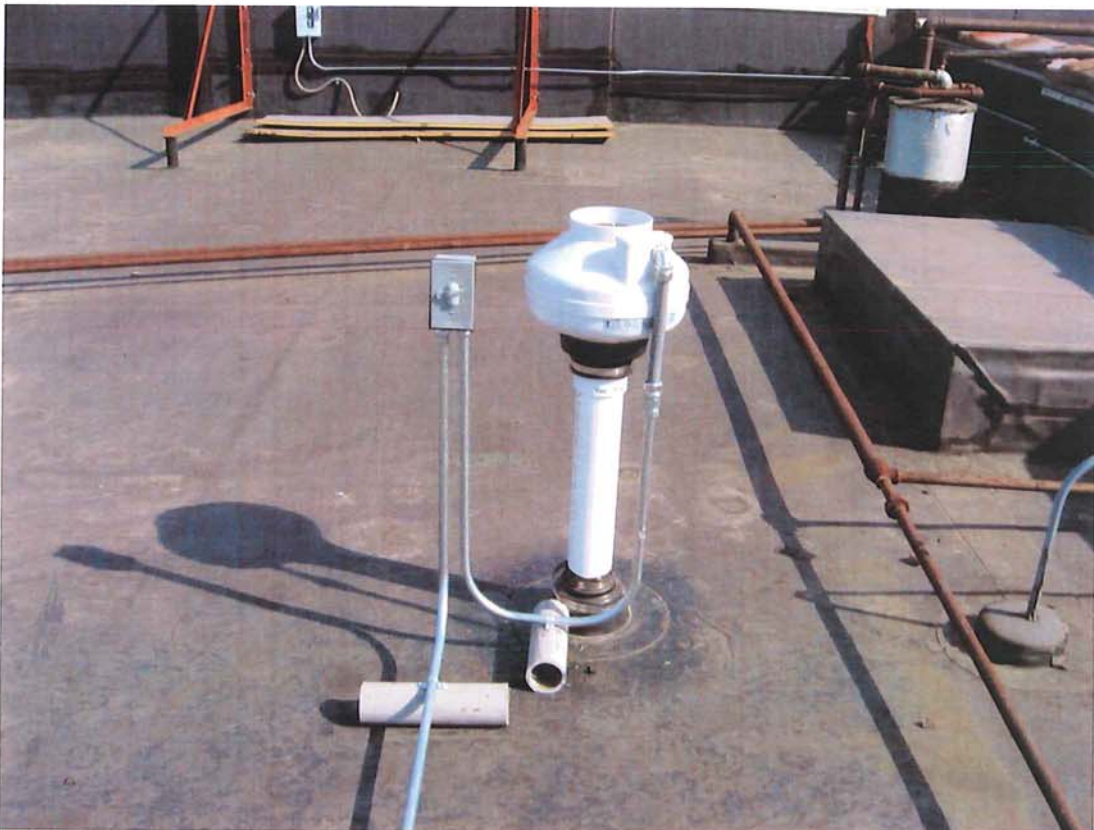
Photograph #: 10 Date: 10/5/2012 Direction: System #4 Subject: Fan mounted on roof with on/off switch
