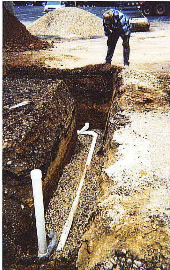
Photo No. 10 - Looking west, picture of the 3-inch manifold piping between Trenches 3 and 4 , and the installation of the north cleanout pipe in Trench 4 (Trench 3 cleanout is visible in the foreground).
