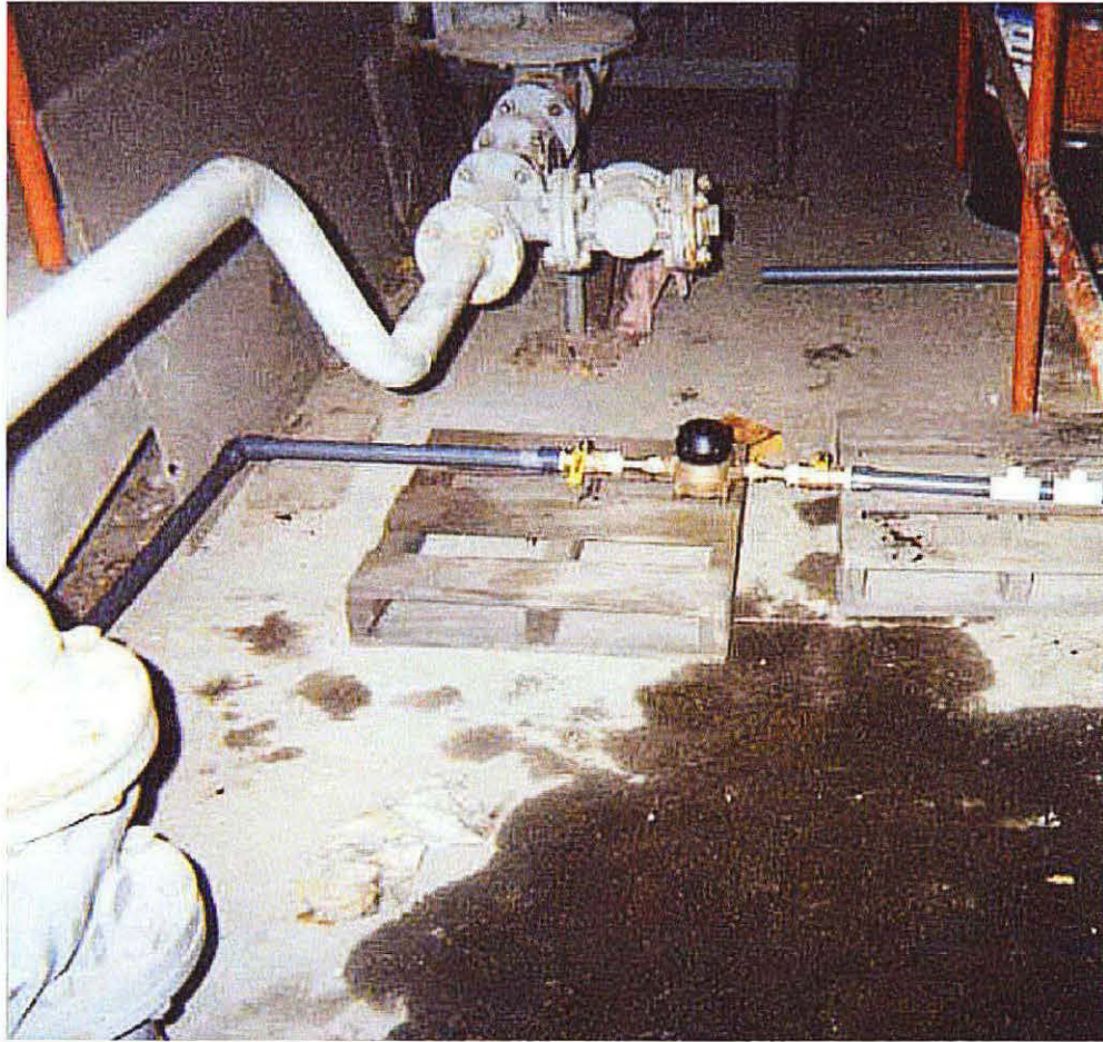
Photo No. 28 - Looking north, picture of the 1-inch-I.D. piping and the water supply flow meter.
