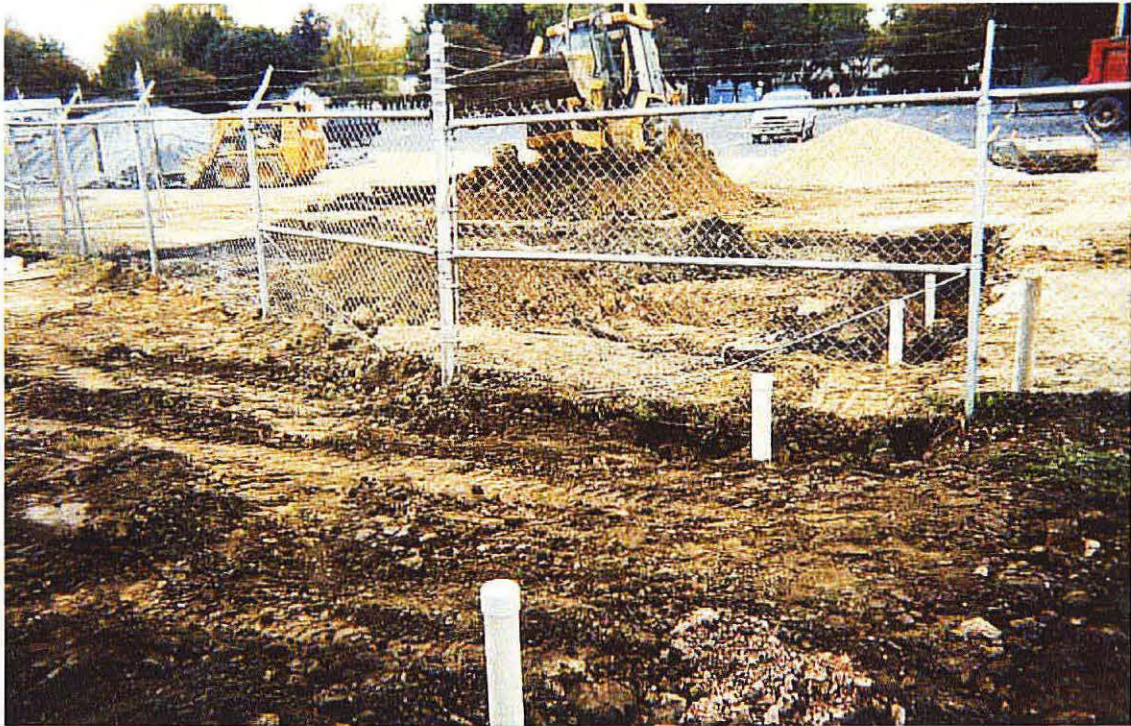
Photo No. 12 - Looking west, picture of the four northern end cleanouts after the manifold piping had been placed and the trenches had been backfilled with clay soil.
