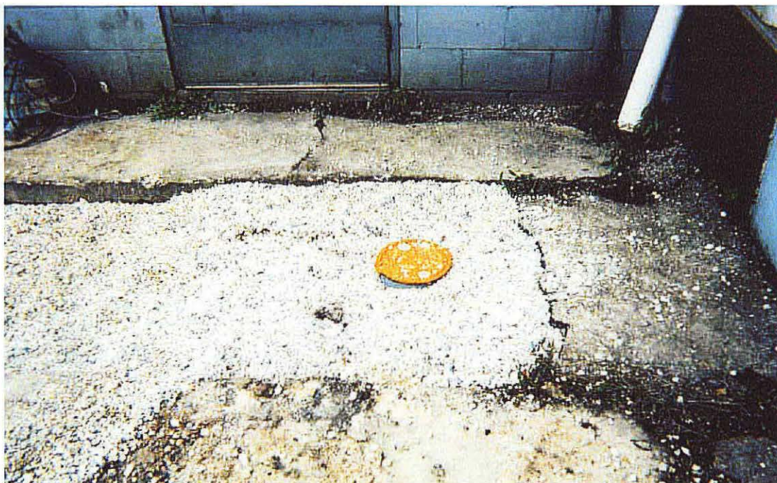
Photo No. 13 - Looking east, picture of heavy-duty flush mount on the southern end cleanout for Trench 1. The trench has been filled to grade.
