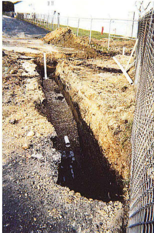
Photo No. 6 - Looking north, picture of Trench 3. A 10-foot segment of perforated pipe has been placed, and the trench has been backfilled with pea gravel.
