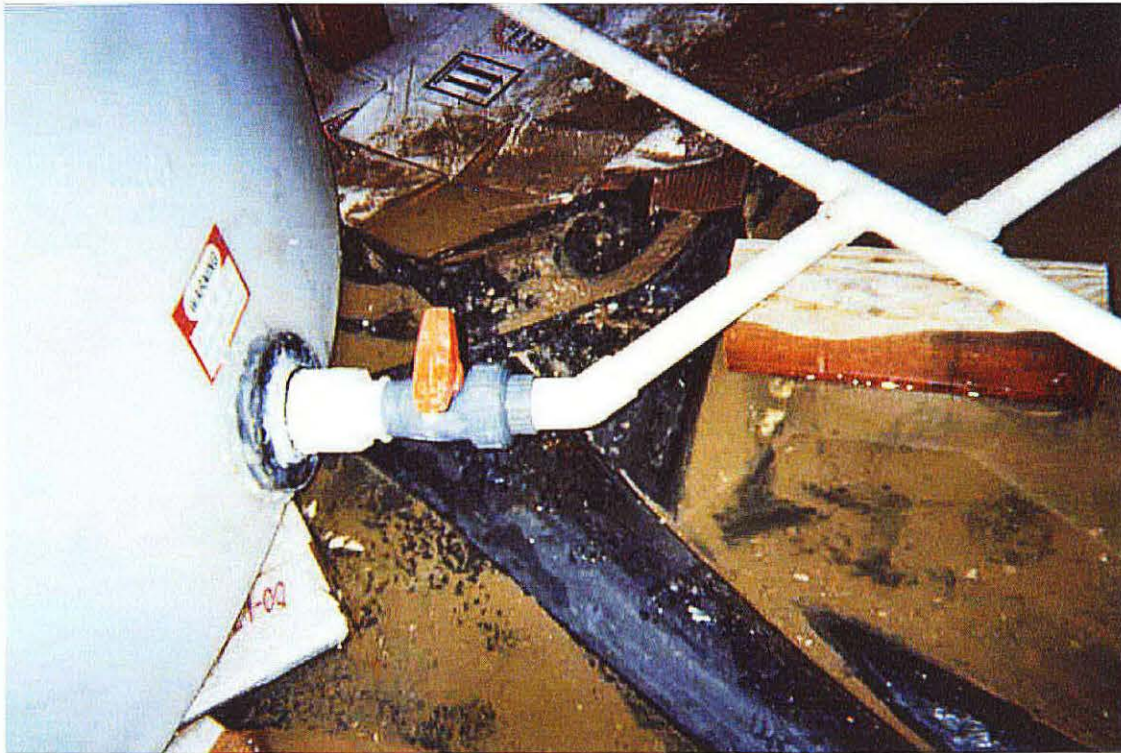
Photo No. 22 - Looking northwest, picture of the plumbing connecting Tank 1 to the manifold piping feeding the infiltration trenches, taken from between the tanks.
