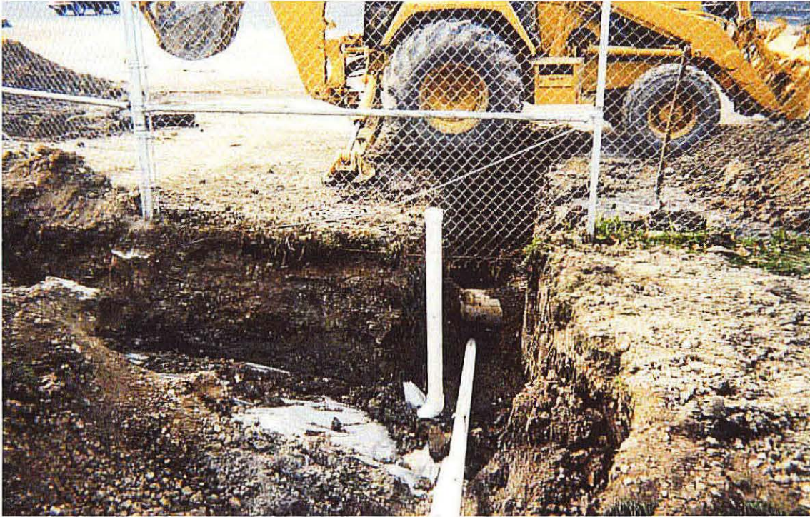
Photo No. 11 - Looking west, picture of the 3-inch manifold piping between Trenches 2 and 3. Manifold pipe was placed under a storm sewer.
