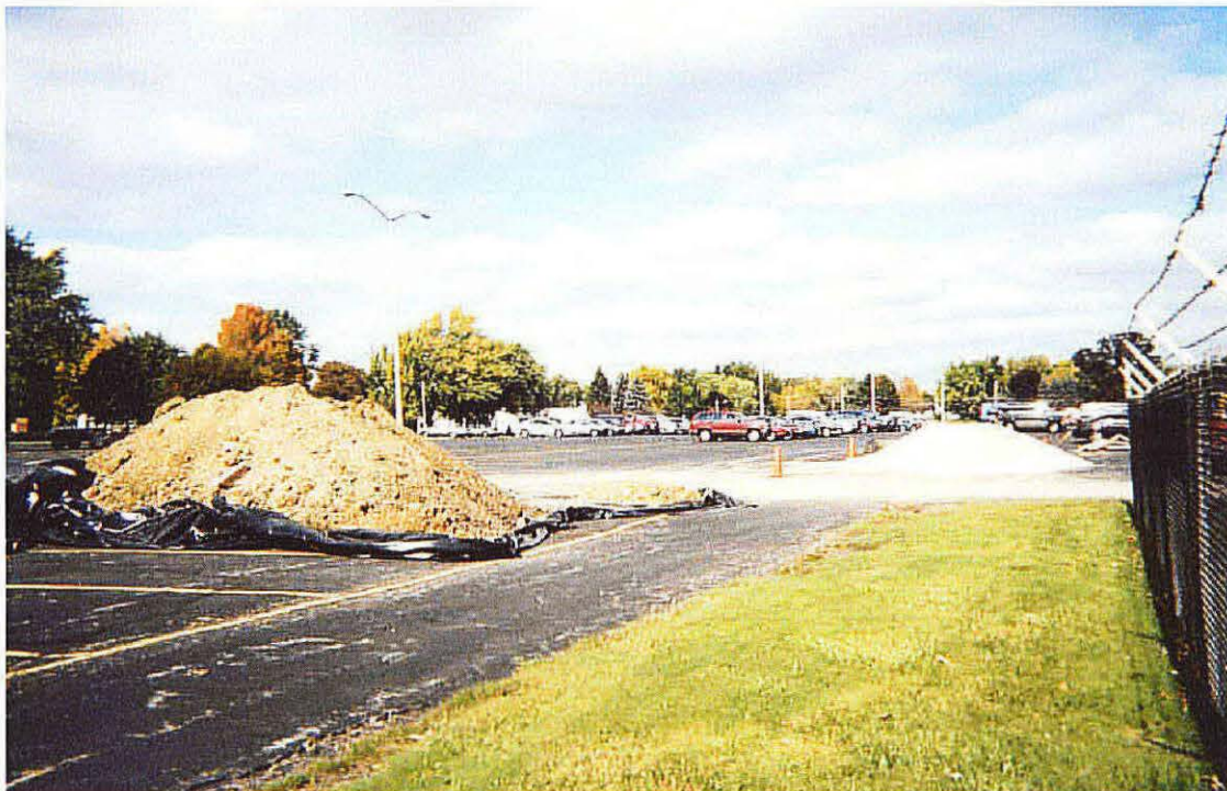
Photo No. 2 - Picture of soil excavated from Trench 1 and 2, stockpiled on 10-mil polyethylene.
