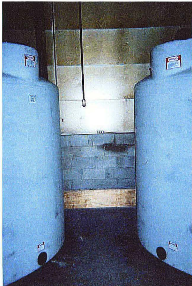
Photo No. 18 - Looking west, picture of the completed spill containment wall and 20-mil liner as viewed from between the tanks.
