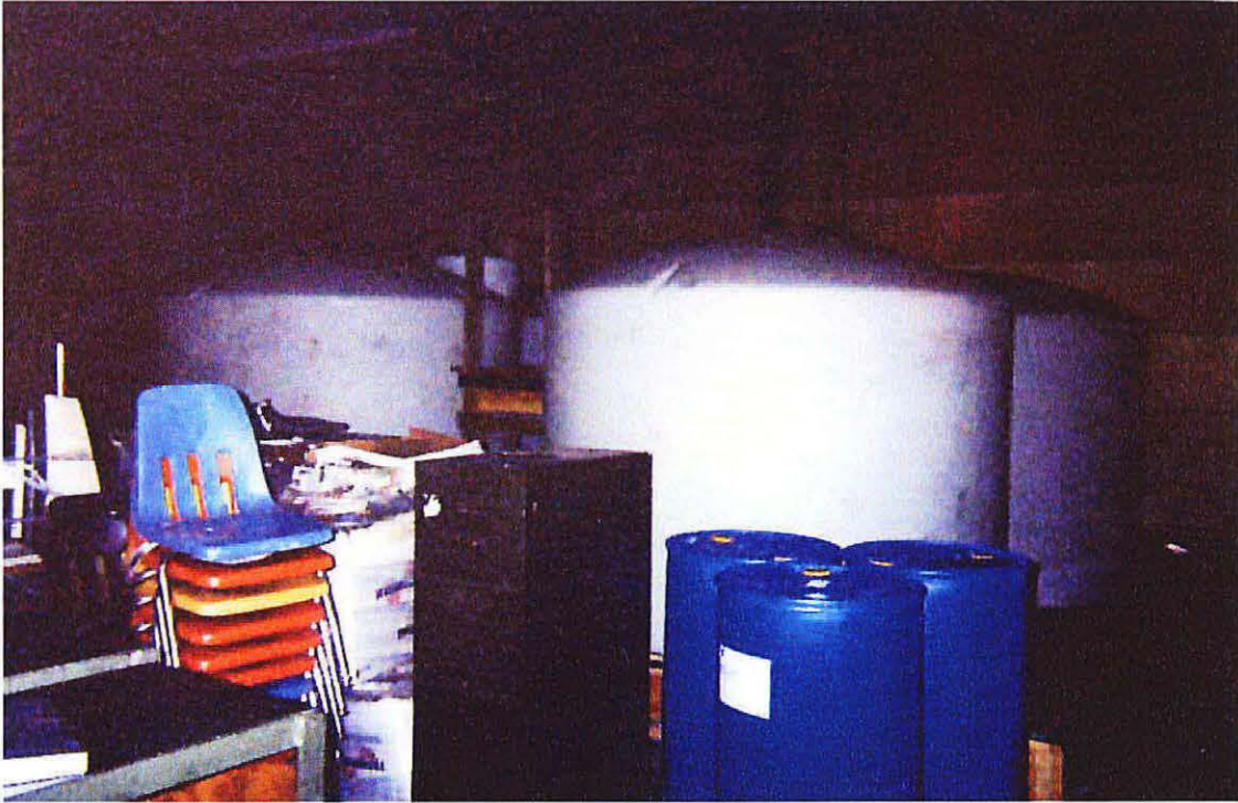
Photo No. 19 - Looking southwest, picture of the four storage tanks after the access platform and ladder construction was completed.
