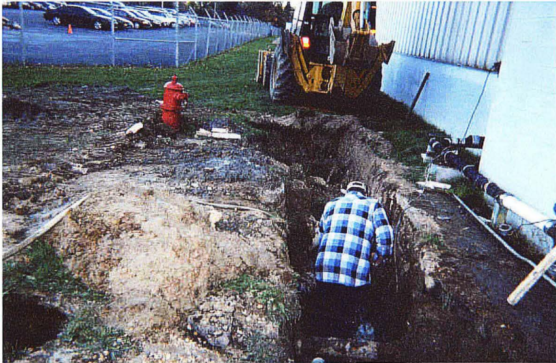
Photo No. 1 - Looking north, picture of the excavation of Trench 1 with a backhoe.
