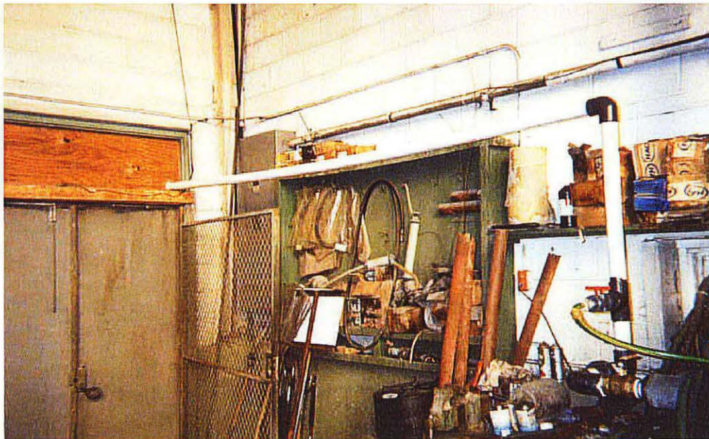
Photo No. 25 - Looking northeast, picture taken inside the Tecumseh facility's boiler room, which shows the plumbing between the pressurized water supply to the location where the 2-inch-I.D. piping exits the building along the southern end of the Recycling Dock Area.
