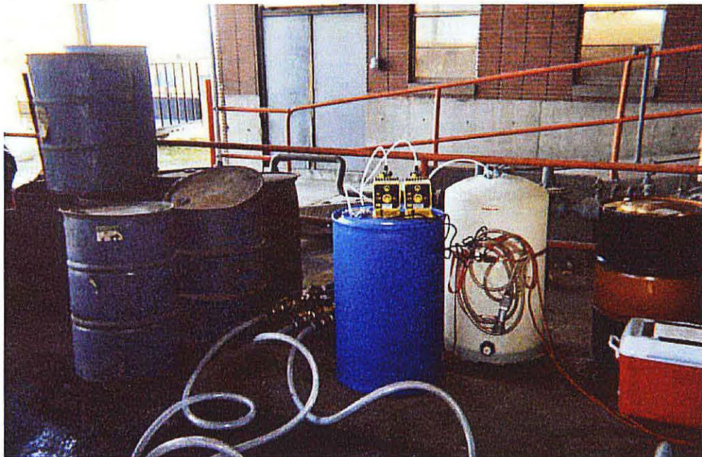
Photo No. 29 - Looking south, picture of the chemical supply system. The drum containing lactate (blue) and the drum containing the remaining reducing agents (white) are shown with the chemical metering pumps (located on top of the blue drum).
