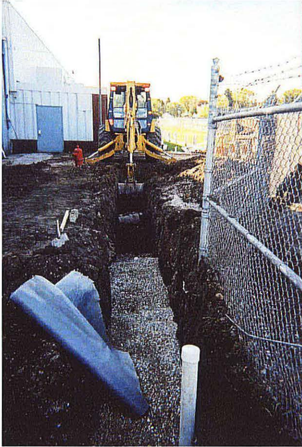
Photo No. 5 - Looking south, picture of the excavation of Trench 2. A 10-foot segment of perforated pipe has been placed, and the trench has been backfilled with pea gravel.
