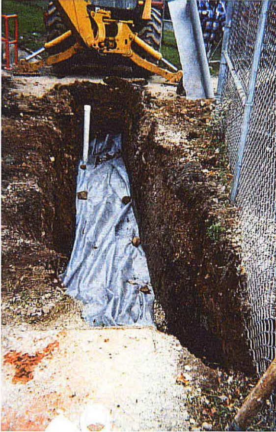
Photo No. 9 - Looking south, picture of Trench 2 after the geotextile filter had been placed on the gravel fill.
