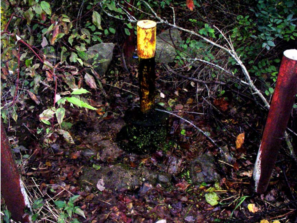
MW7B. View showing continued water seepage following installation of well plug to 4' below grade.
