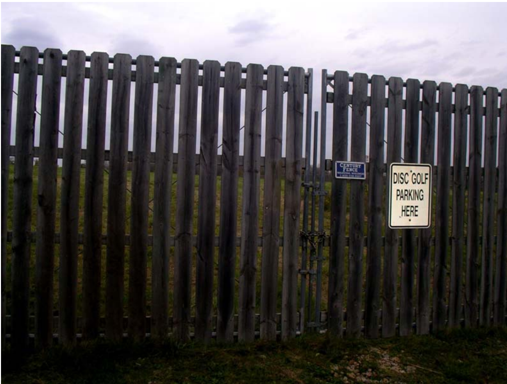
Front gate at the end of Amundson Parkway showing missing front gate sign.
