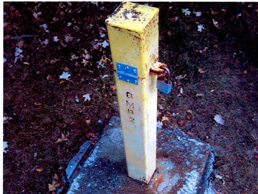
2012-09-012: GMP-2 – New Hinge Installed Date: 01-Oct-2012 Time: 5:50 PM Weather: P-Cloudy, 65 Degrees F.
