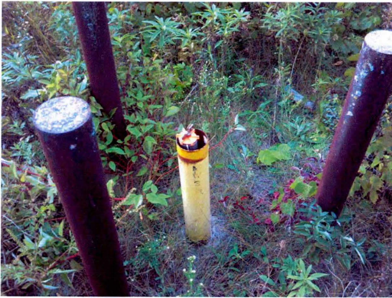
2012-09-013: MW-3S - New Well Cap Installed Date: 19-Sept-2012 Time: 9:48 AM Weather: Partly Cloudy, 65 Degrees F.
