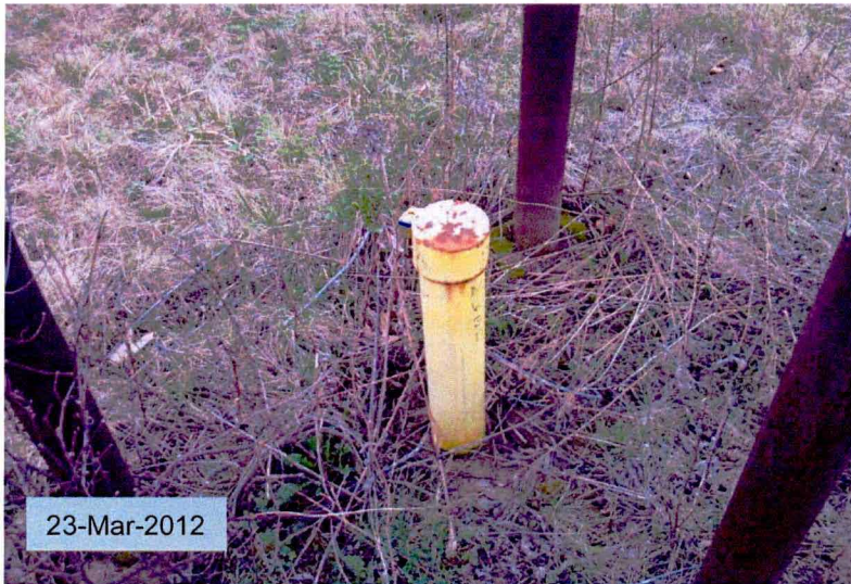
2011-10-007 : MW-3D lock was damaged and replaced during inspection.
