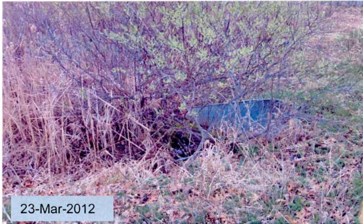
2011-10-029 : Woody vegetation in front of culvert in south drainage feature.
