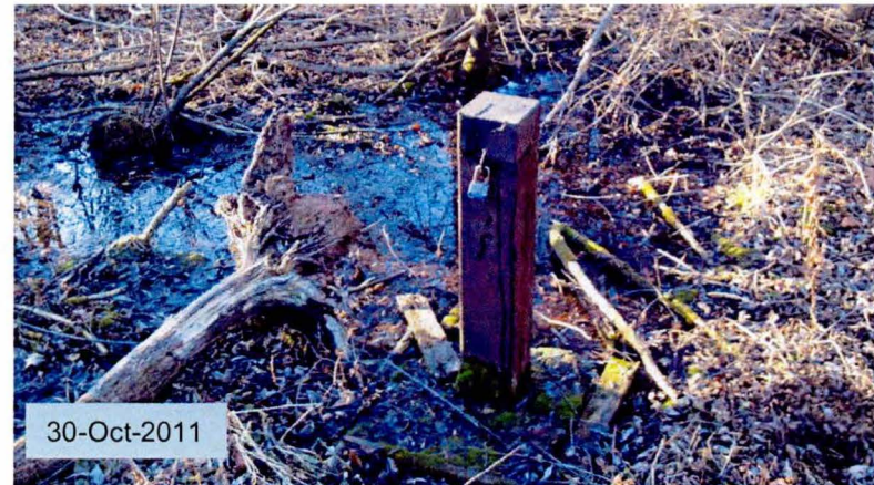
2011-10-012 : MW-10D – Well is self-purging and requires plugging.
