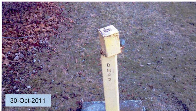
2011-10-023 : GMP-2 protective casing requires a new hinge.
