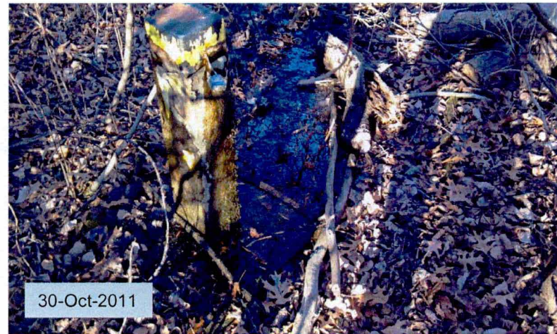
2011-10-020 : OW-1 is self-purging, showing signs of flowing at the concrete well foundation. Requires plugging. Lock was damaged and required replacement.
