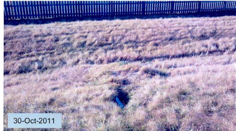
2011-10-002 : Erosion feature on northwest area of cap near GV-18 (Top View).
