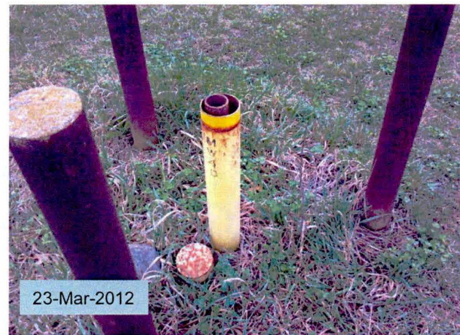
2011-10-008 : MW-4D requires a new 2-inch expandable cap.
