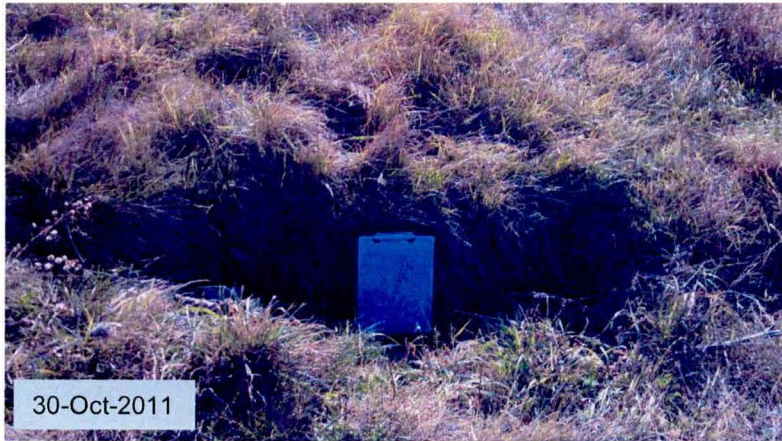
2011-10-001 : Erosion feature on northwest area of cap near GV-18 (Side View).
