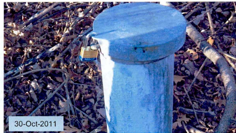
2011-10-022 : EW-1 lock was missing and required replacement
