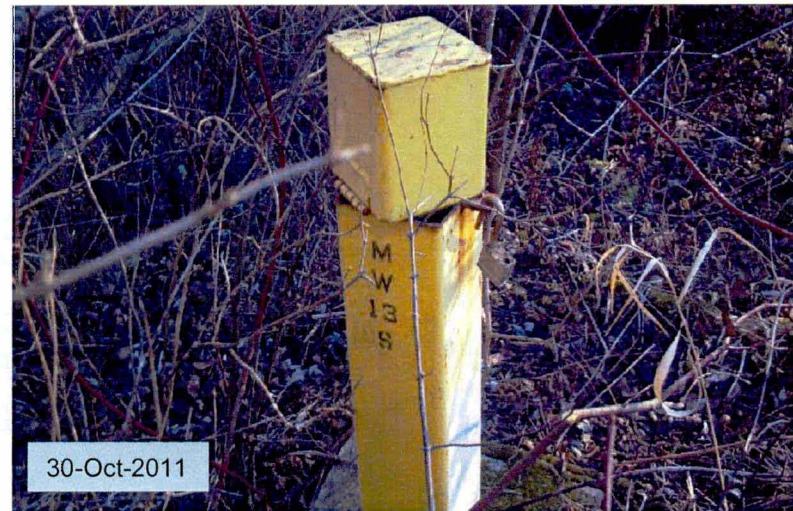
2011-10-016 : MW-13S protective casing requires a new hinge.
