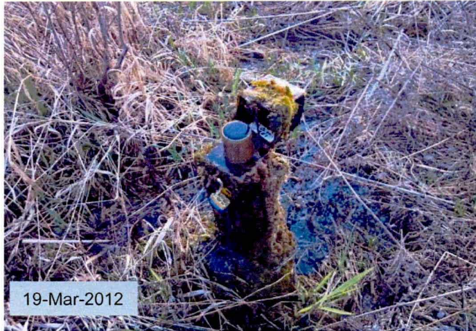
2011-10-017 : MW-13D protective casing is covered in moss. Lock was damaged and replaced. Well is self purging.
