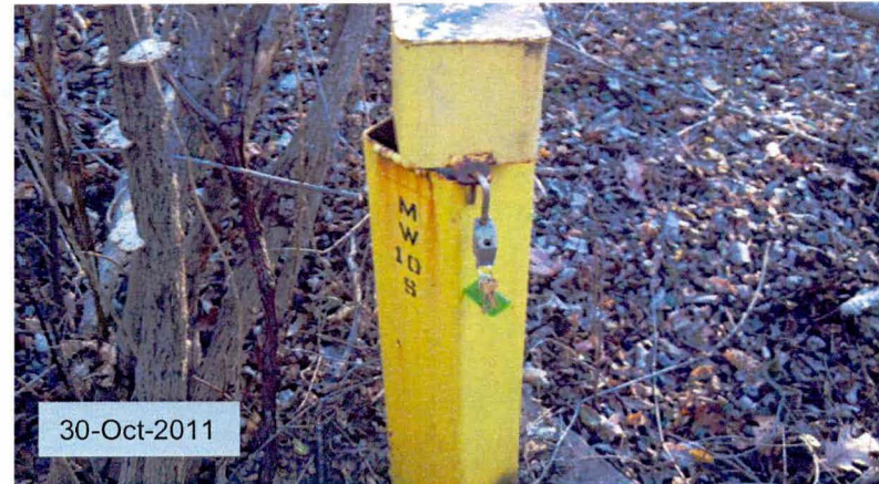
2011-10-014 – MW-10S protective casing requires a new hinge.
