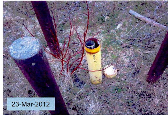
2011-10-006 : MW-3S requires a new 2-inch expandable cap.
