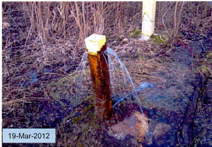
2011-10-015 : MW-13I is self-purging and requires plugging. Lock was damaged and required replacement.
