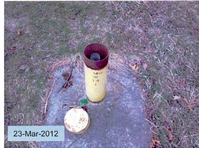
2011-10-018 : MW-14I requires a new two-inch expandable cap.
