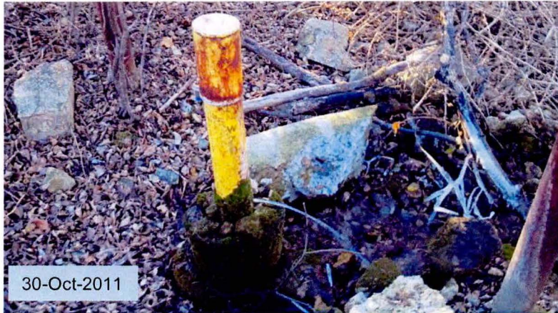
2011-10-009 : MW-7B is flowing through weep hole and requires plugging. Lock was also replaced.
