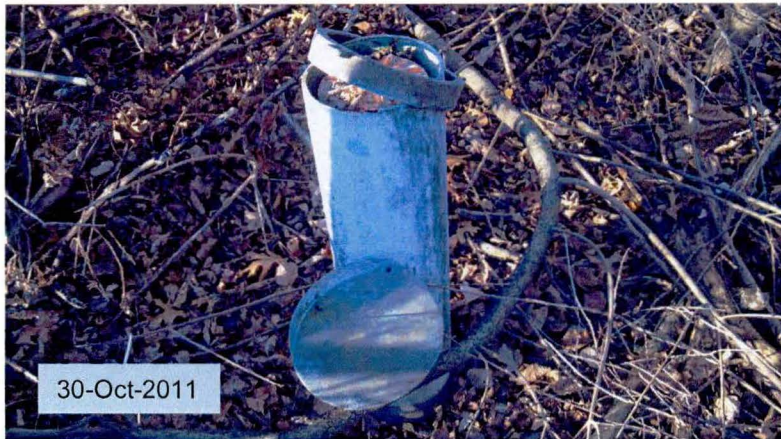
2011-10-021 : EW-1 locking ring at the top of casing requires repair.
