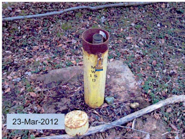
2011-10-019 : : MW-15D requires a new two-inch expandable cap. Lock was damaged and required replacement.
