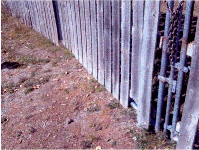
2012-10-001: Broken and warped slats on south access gate
