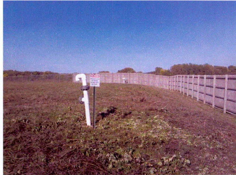
2012-10-020: GV-1 – Landfill Cap After Mowing Date: 15-Aug-2012 Time: 3:45 PM Weather: Sunny, 80 Degrees F.
