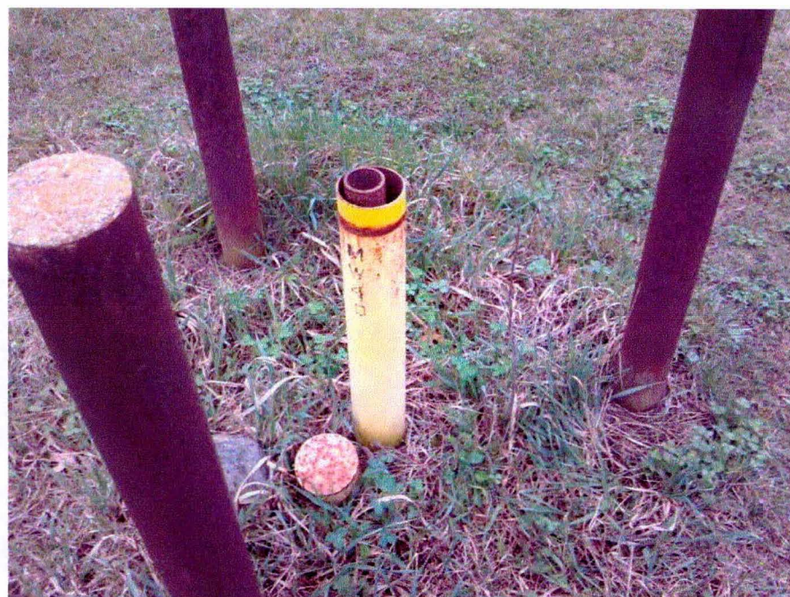
2012-10-014: MW4D – Well casing too high to allow installation of expandable cap Date: 23-Mar-2012 (Historical photo) Time: 2:49 PM Weather: Sunny, 35 Degrees F.
