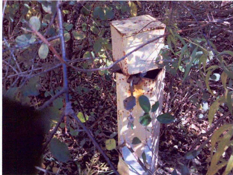
2012-10-018: MW-13S requires new hinge
