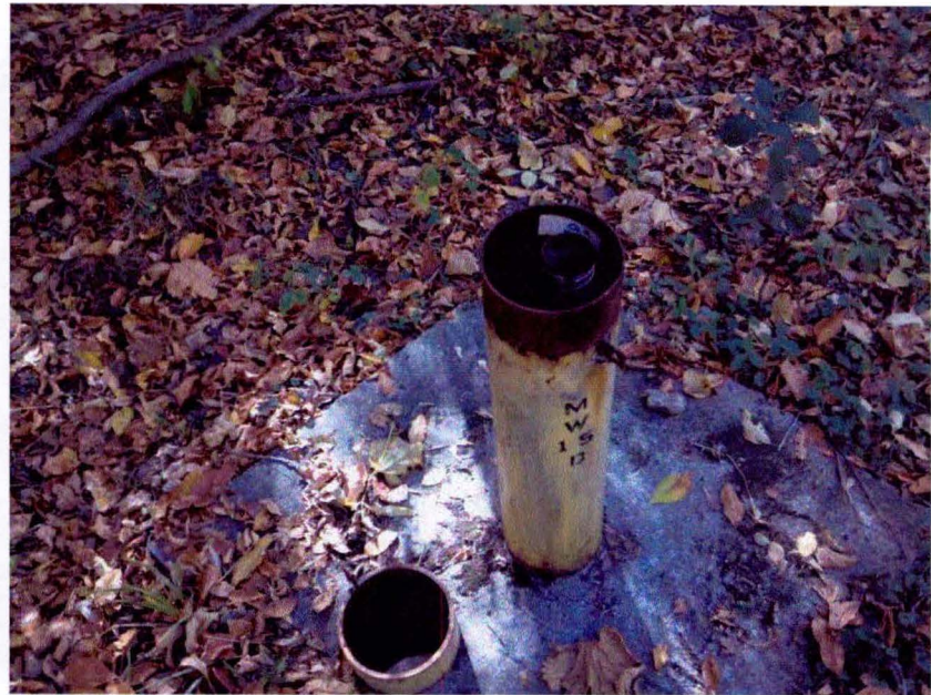
2012-10-016: MW15D – Well casing too high to allow installation of expandable cap Date: 12-Oct-2012 Time: 1:53 PM Weather: Sunny, 50 Degrees F.
