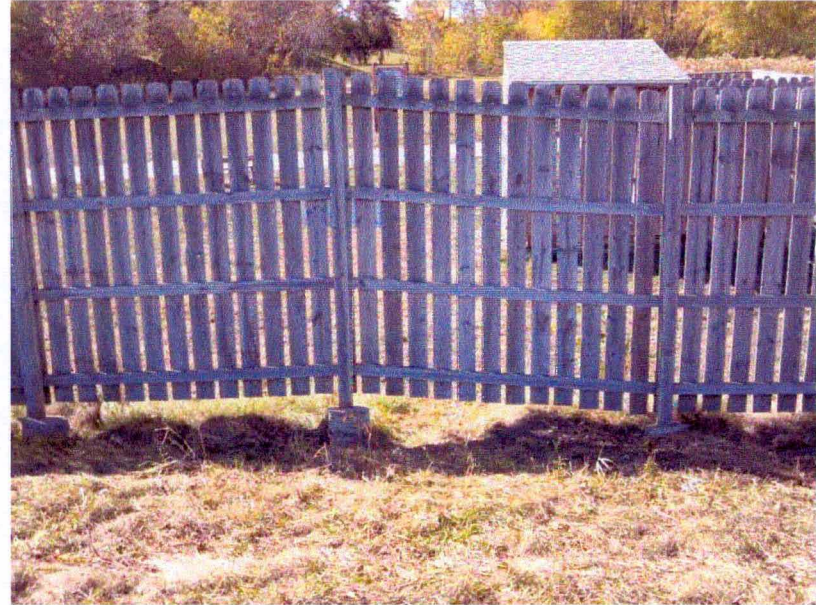
2012-10-002: Frost heave has lifted fence at SW perimeter.
