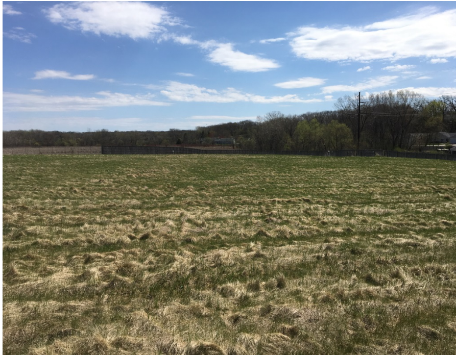
Photo 1: Photo facing east just inside the west access gate. Final cover was damp but in good condition.
