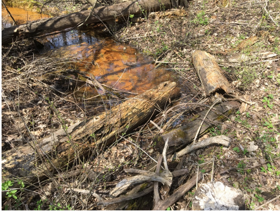
Photo 9: Photo facing southeast. Debris restricting flow in a culvert on the north side of the property near the MW-13 cluster.
