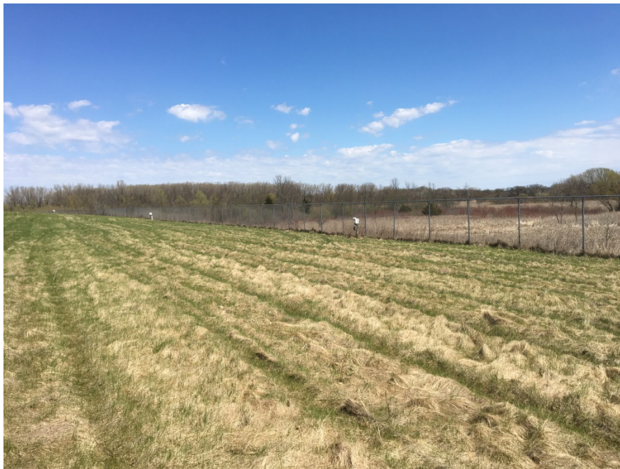
Photo 2: Photo facing northeast just inside the south access gate. Final cover was damp but in good condition.
