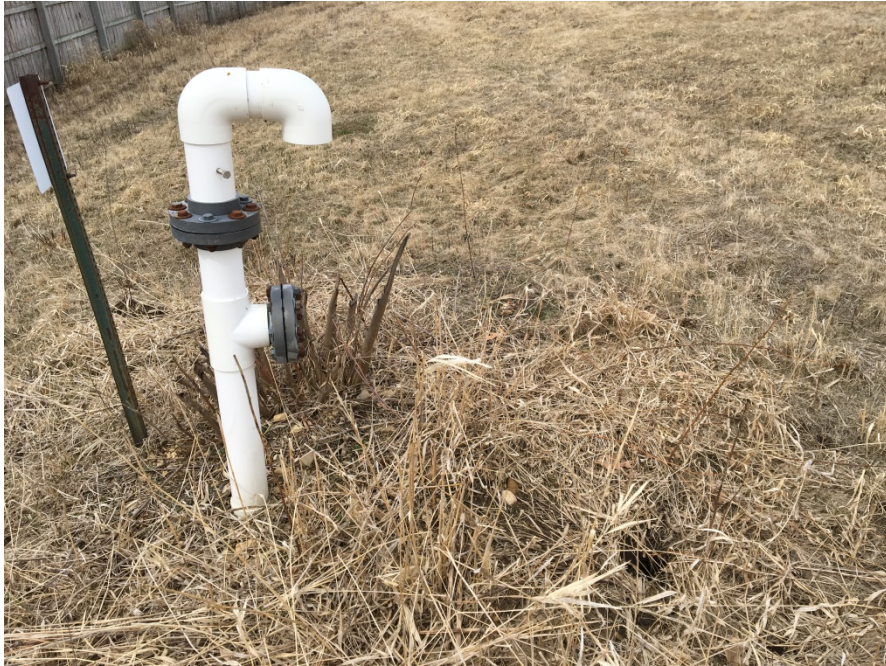
Photo 3: GV-11 is functional but missing an identification label (looking west).
