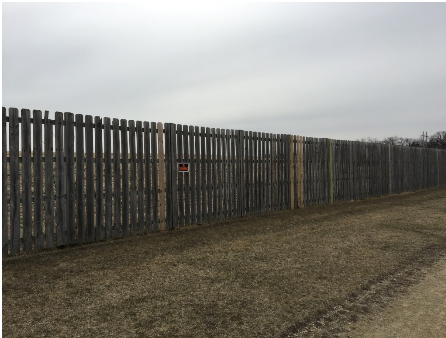
Photo 6: West perimeter security fencing depicted; slats were recently replaced and new signage “NO TRESPASSING” was posted (Looking southeast).
