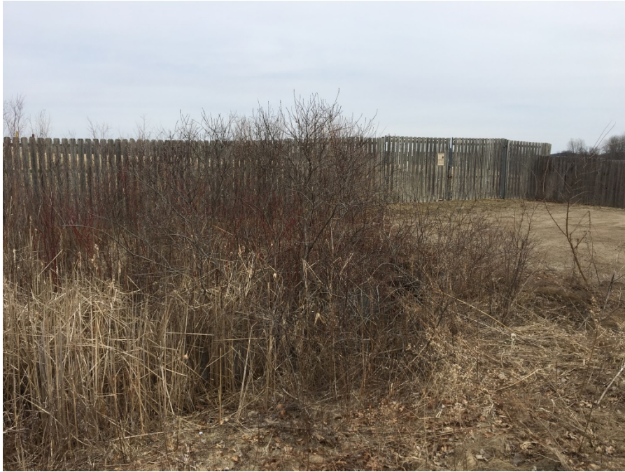
Photo 5: Large shrubs inhibiting water flow into culvert near the south gate entrance (looking northeast).
