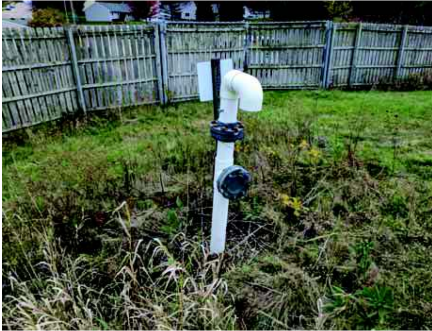
Photo 3: GV-1 is functional but is missing an identification label (Looking south)
