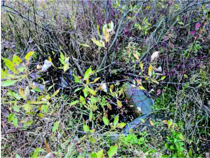
Photo 5: Large shrubs inhibiting water flow into culvert near the south gate entrance (Looking west)
