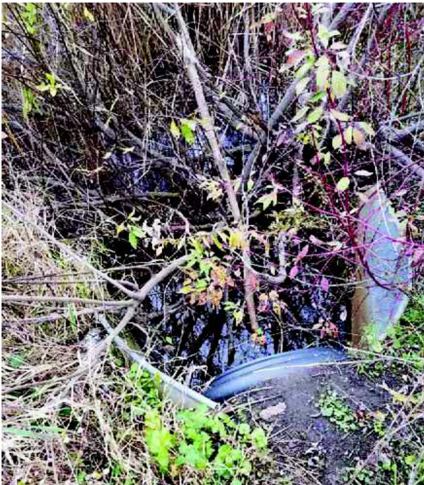
Photo 18: View west toward west end of culvert near Main Gate. Drainage channel partially blocked with branches.
