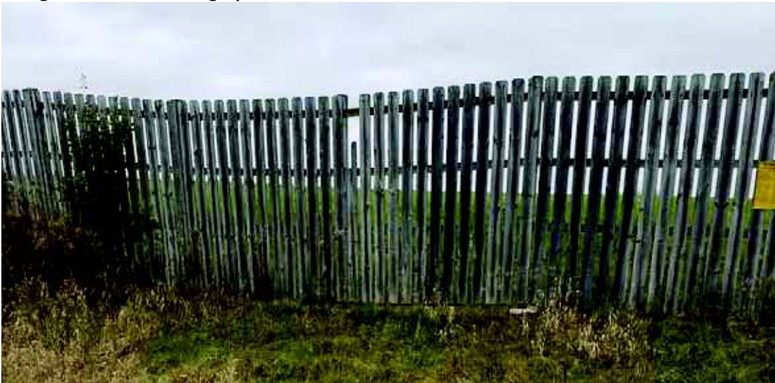
Photo 17: View east toward broken slat on west fence line.
