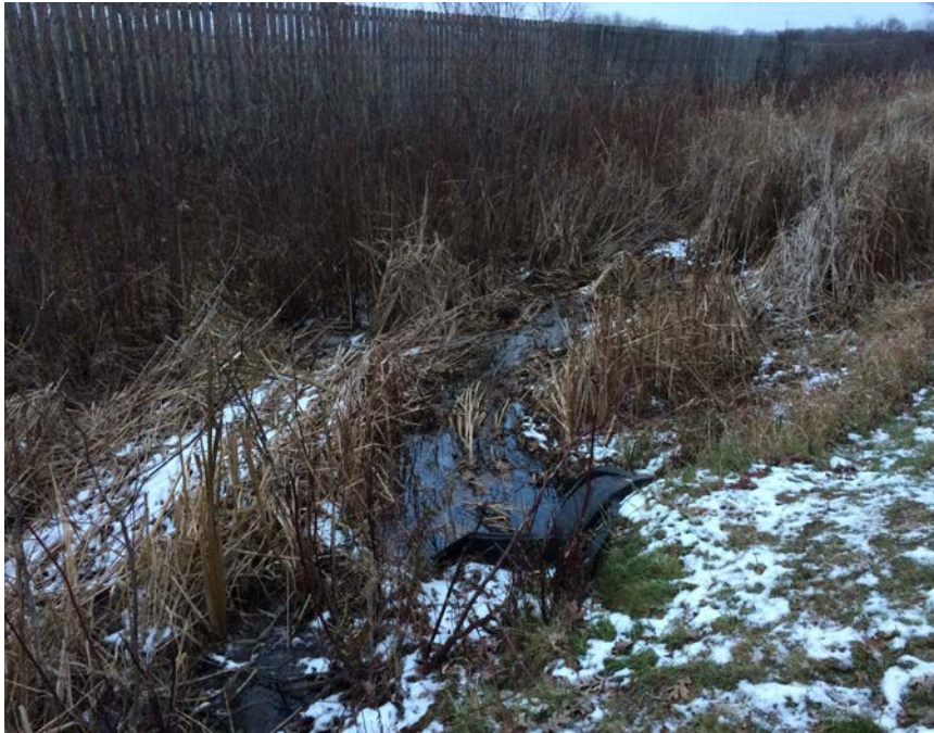
Photo 1: Vegetation by culvert on south side of landfill.
