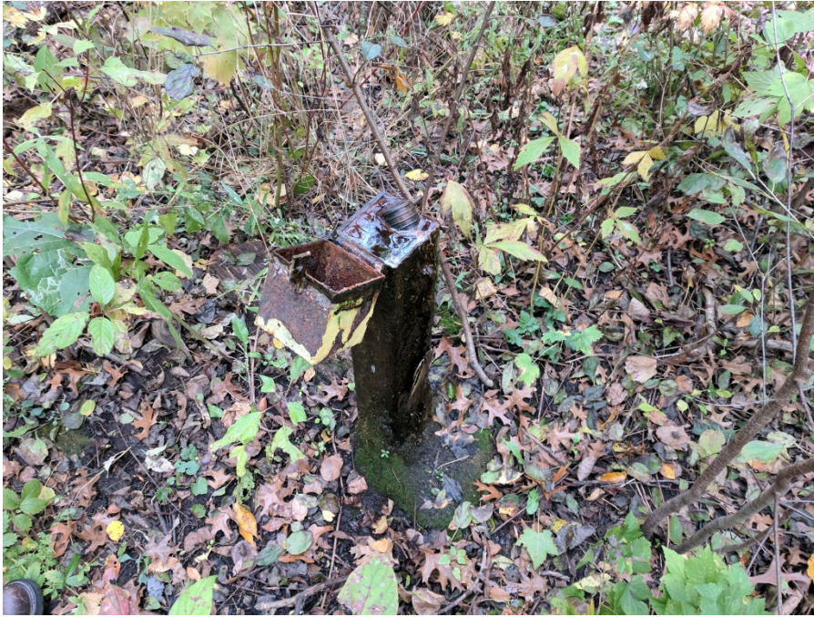
Photo 7: OW-2 casing flooded with water, well plug was floating (Looking down)
