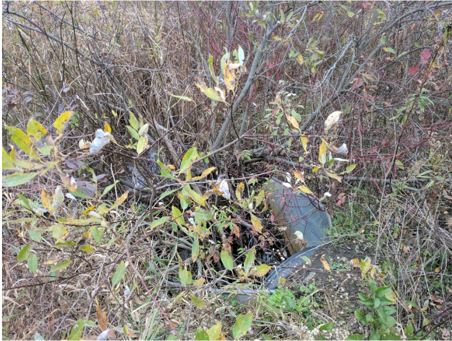
Photo 5: Large shrubs inhibiting water flow into culvert near the south gate entrance (Looking west)
