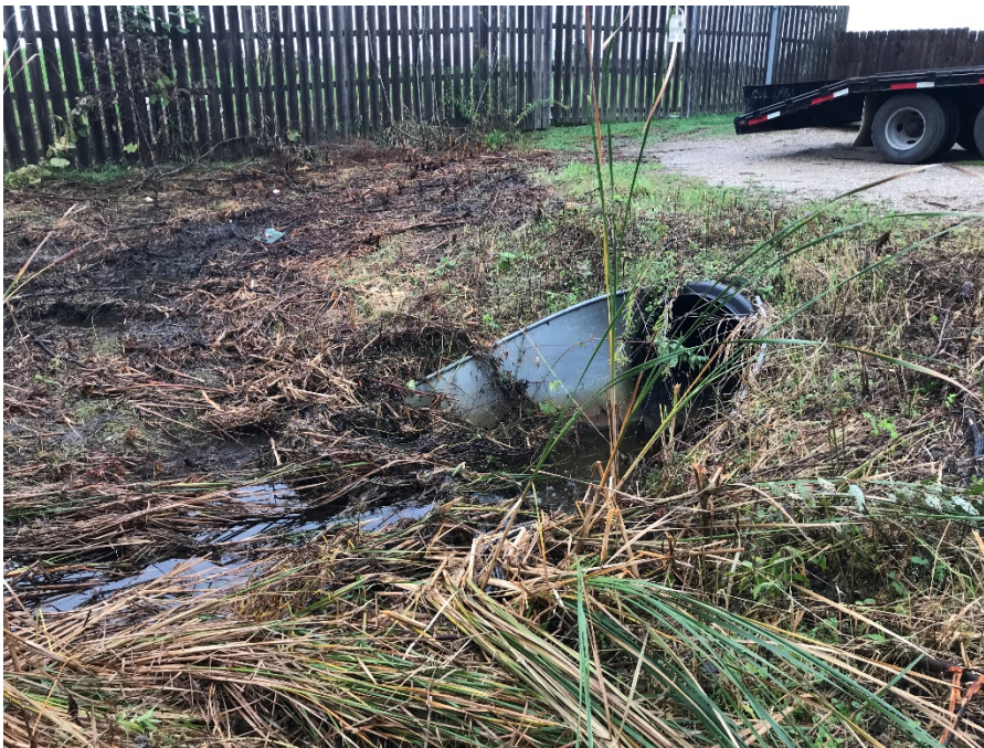
Photo 2: View of culvert outside of southeast gate recently cleared of vegetation (looking northeast).
