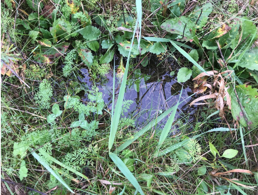
Photo 1: Slight surface water ponding on landfill cap after recent storm events (looking down).
