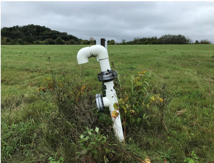
Photo 4: GV-8 slightly out of plumb, though apparently functional (looking west).
