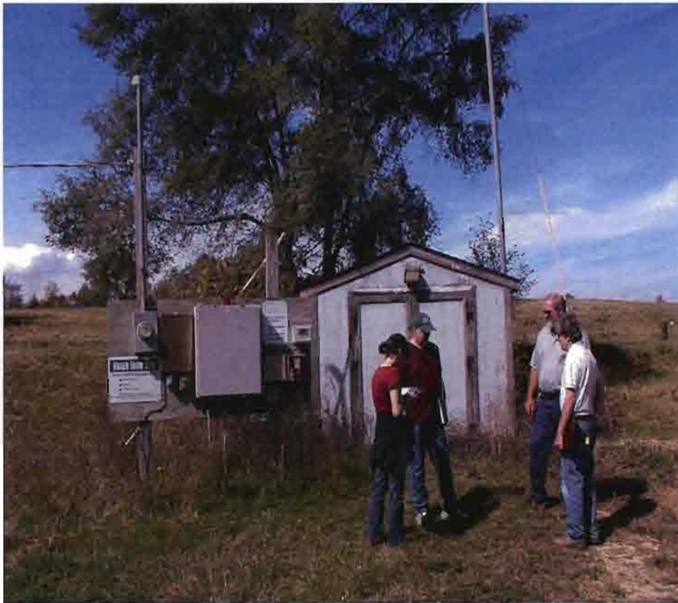
Photo 19 – Facing northwest, view of In-situ vapor extraction (ISVE) shed. The electrical panel is visible to the left of the shed.
