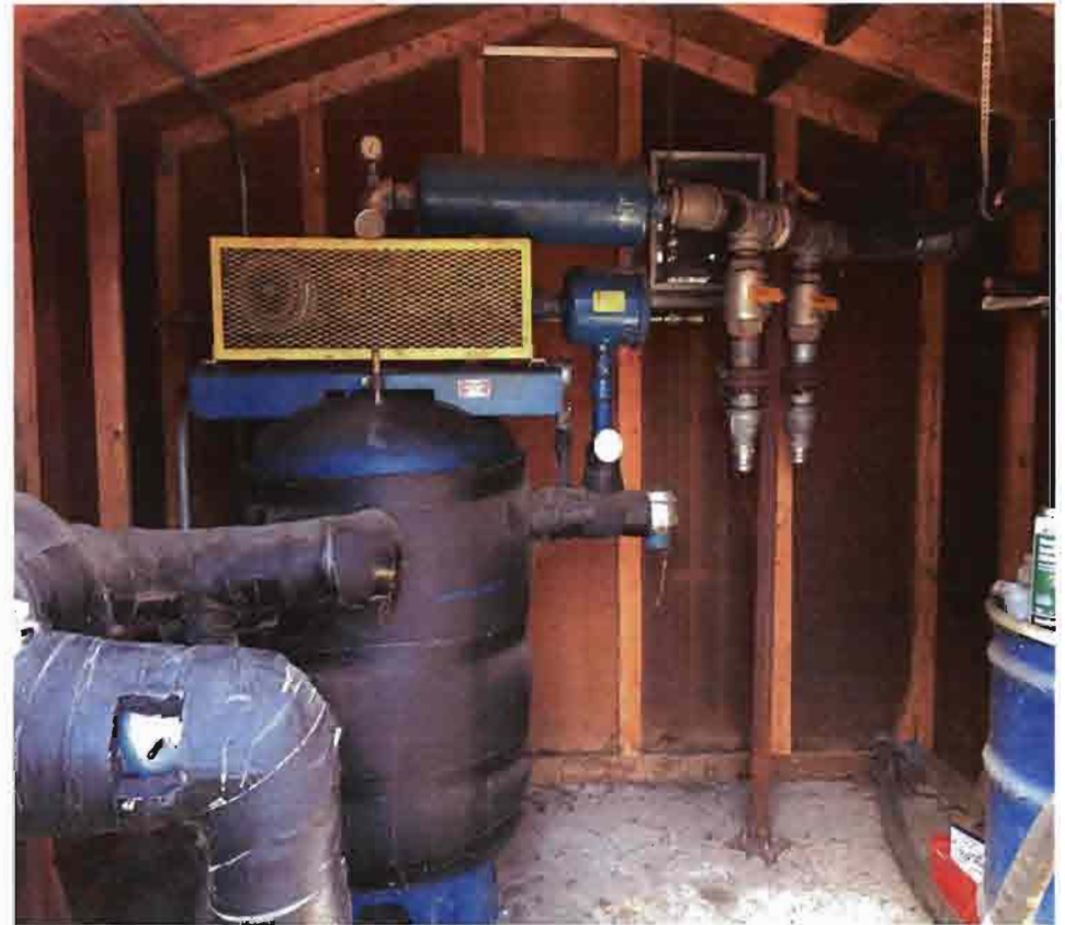
Photo 20 –A view inside the ISVE shed containing the ISVE system blower (back wall) and inlet manifold (black piping in left foreground of photo). The sample port of the inlet manifold is visible in the bottom left foreground.
