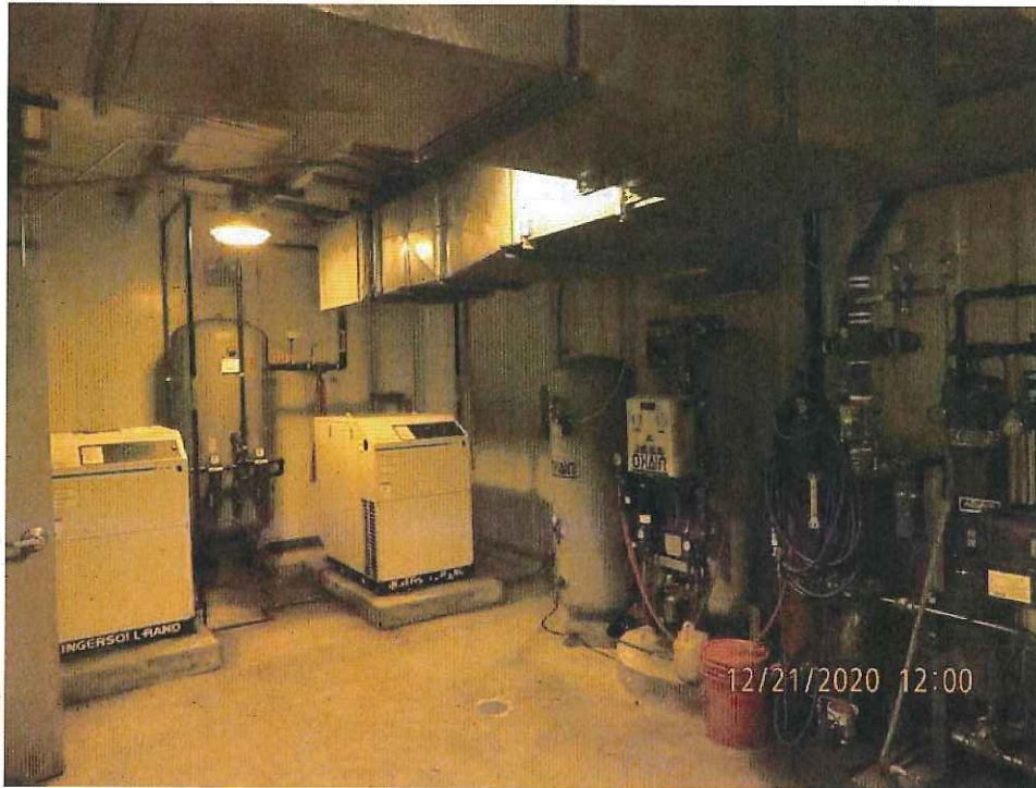
Photo 3: LFAS Components – Air Compressors, Oxygen Concentrator, Air Dryer
