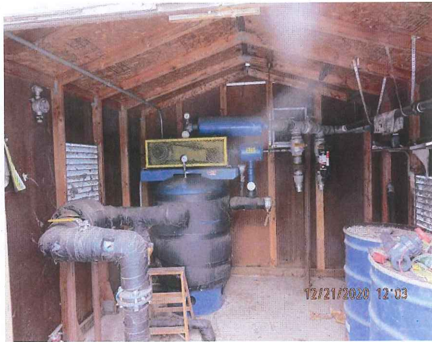
Photo 5: SVE Blower and Header Piping
