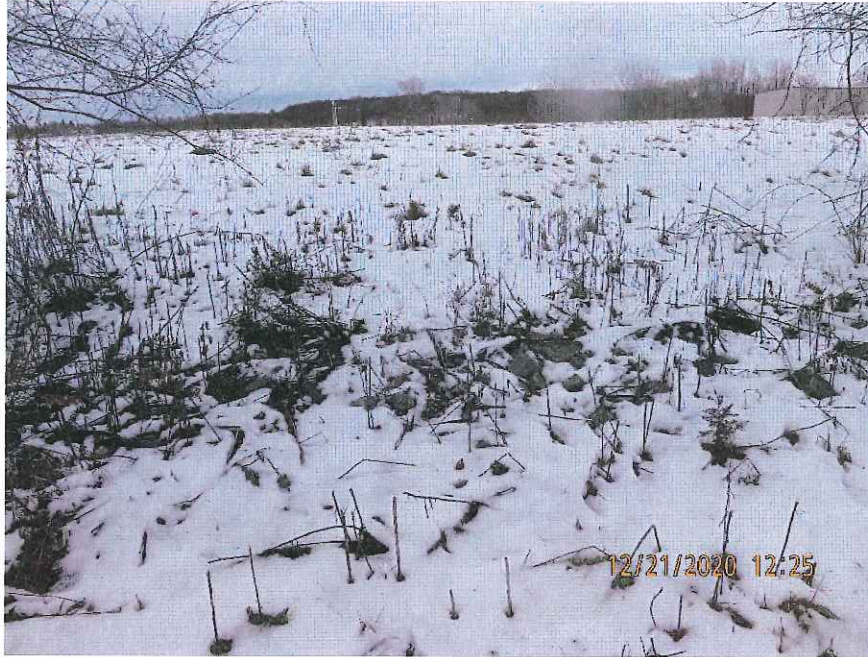
Photo 15: Rip-rap installed as part of the drainage layer of the landfill cap. View looking to the east from the west edge of the cap.
