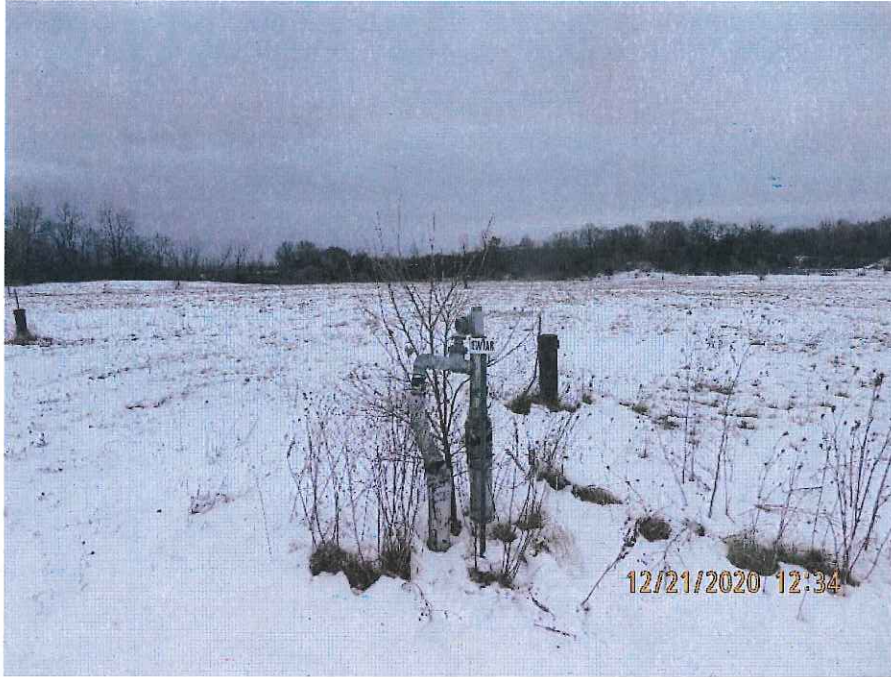
Photo 19: SVE well EW1AR, open to atmosphere to promote air flow into the waste mass. View is to the north from atop the landfill cap.
