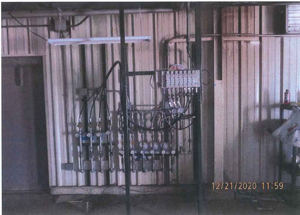
Photo 2: Low Flow Air Sparge (LFAS) Manifold
