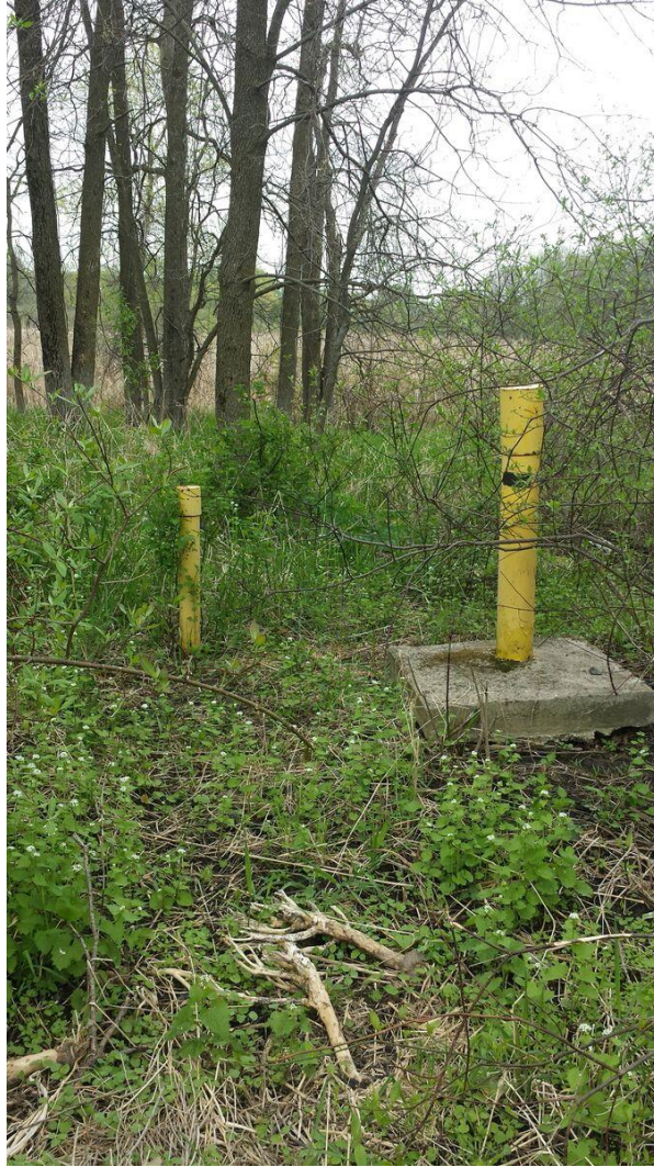
Left: MW-13D Right: MW-13S showing heaved concrete pad.
