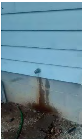
Photo #29 Private Well PW-08 (W2603 Elm St.)
