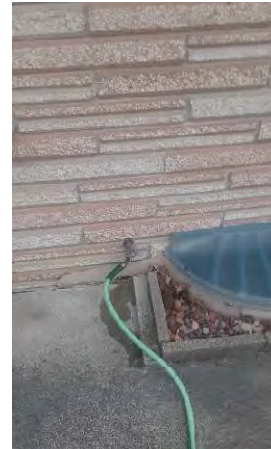
Photo #30 Private Well PW-09 (W2606 Elm St.)
