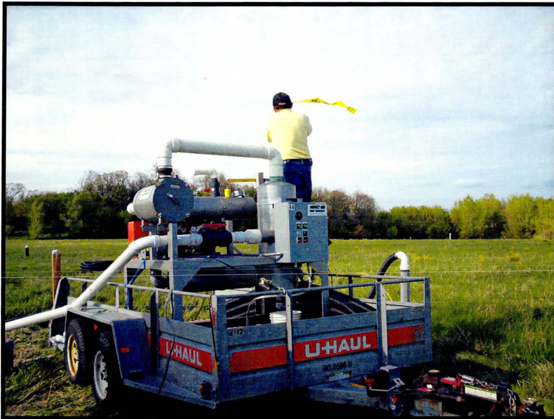
Blower system with control panel (grey box) – looking north-northeast
