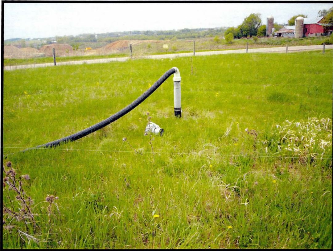
Extracting from gas vent GV-4 – looking northwest
