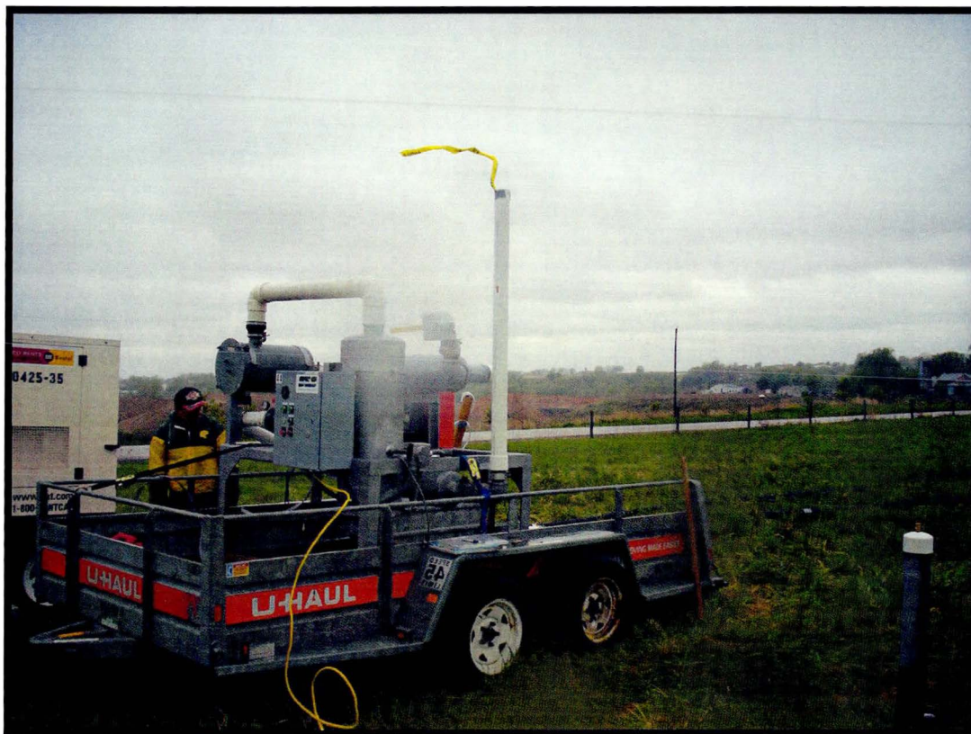
Blower system (looking northwest)
