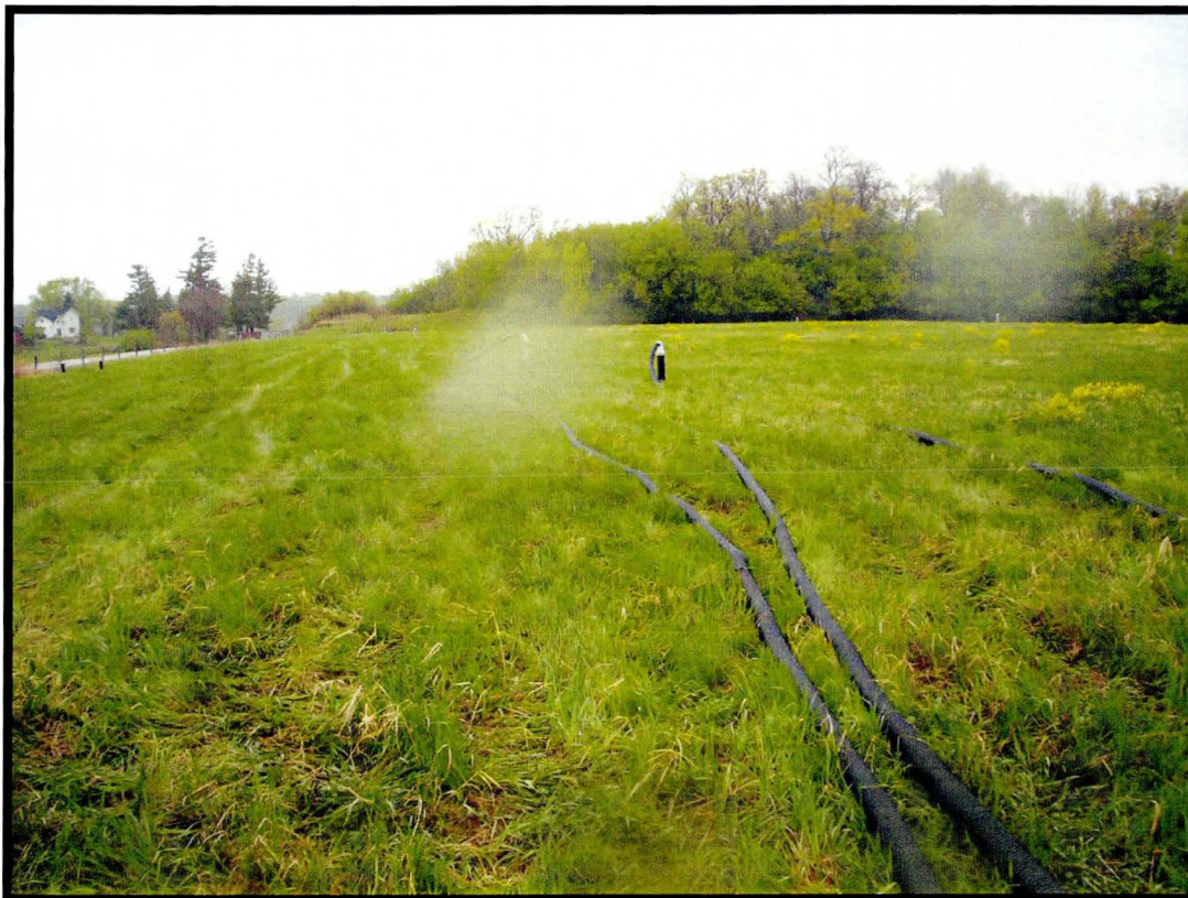
Extracting from leachate well LC-3 and gas vent GV-2 (also extracting from GV-4 to the north)
