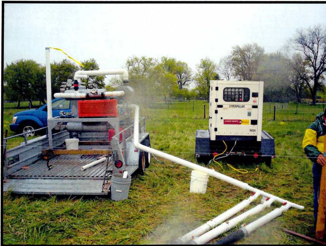
Blower system with system piping/control valves and diesel generator (on right) – facing south
