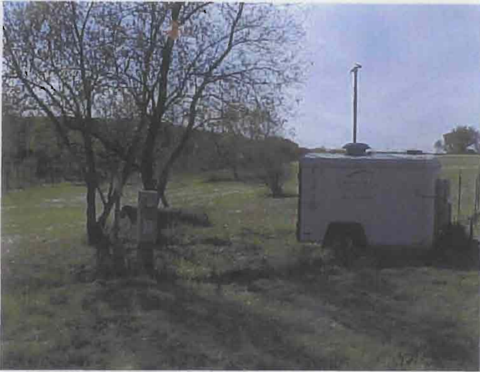
Photo 17 Electrical meter and blower trailer
