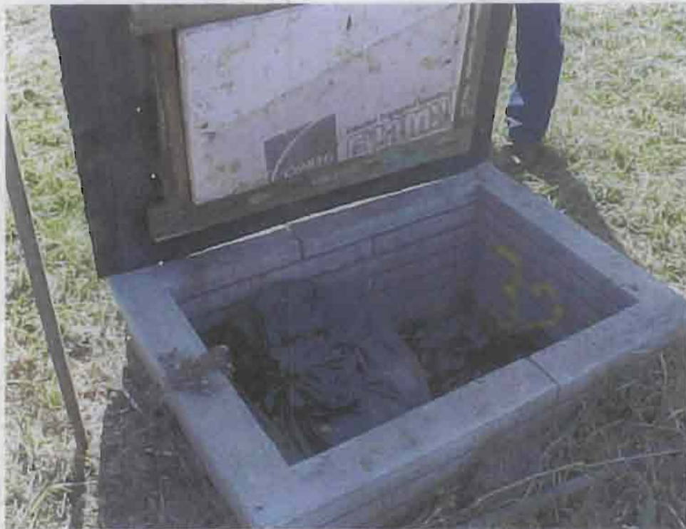
Photo 15 Manifold box with insulation added in bags and on underside of cover
