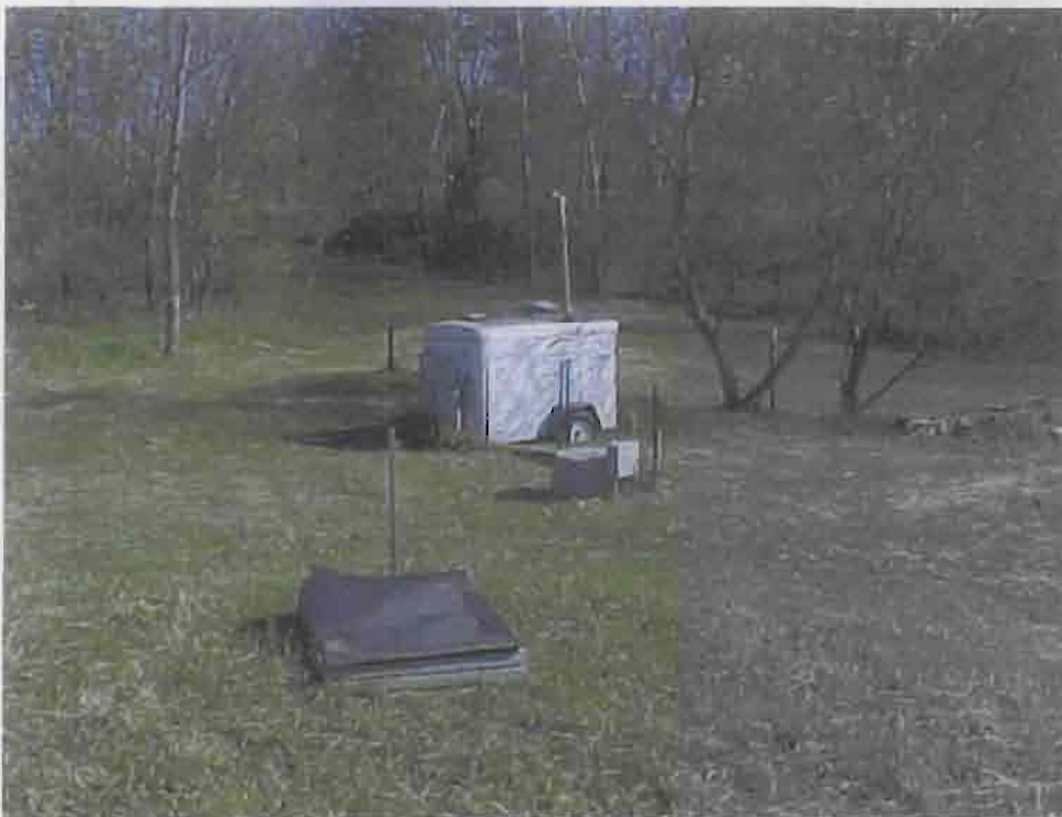
Photo 14 Active gas venting equipment; foreground is manifold box then behind that is the drip tank then behind that blower system trailer
