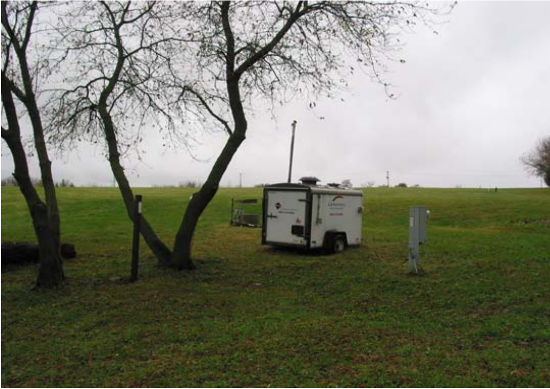
Photo 3 Looking NW towards gas extraction blower trailer
