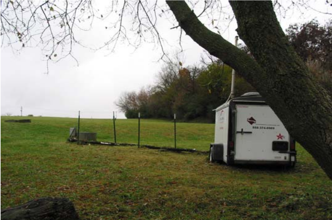
Photo 4 Looking W towards active gas venting equipment; background drip tank, foreground is blower system trailer
