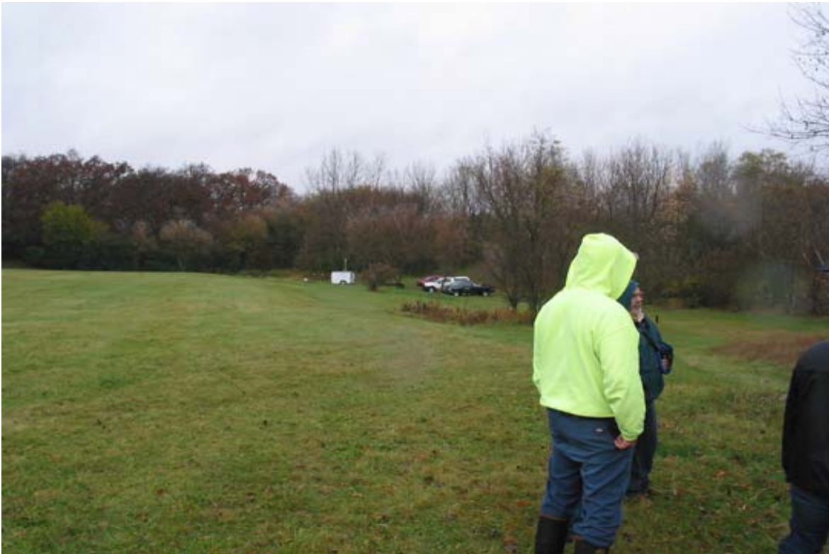
Photo 14 Looking N towards gas extraction equipment from SE corner of LF
