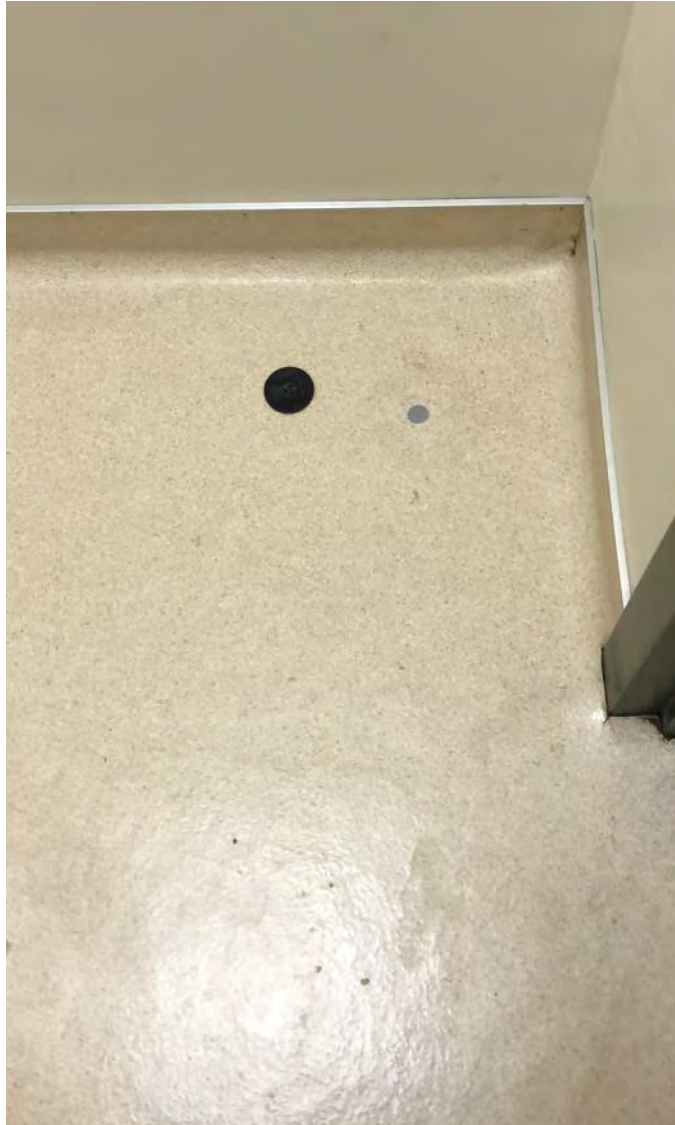
Photo 5: Abandoned temporary vapor point and installed and capped flush mount vapor point VP-8
