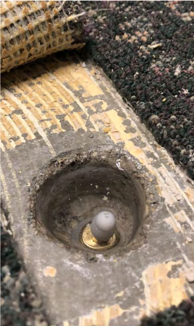
Photo 3: Installed flush mount vapor point VP-4-2R
