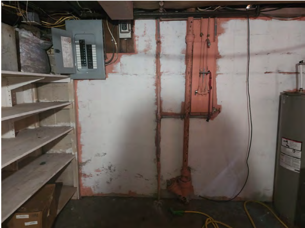
Backroom sewer pipe
