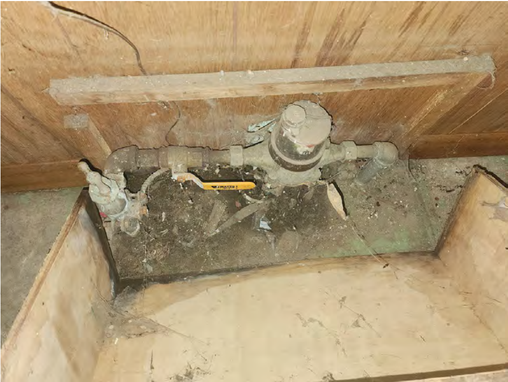
Pipe by stairs
