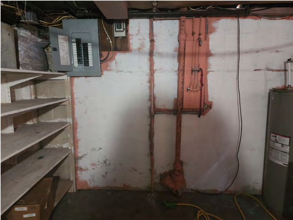
Backroom sewer pipe
