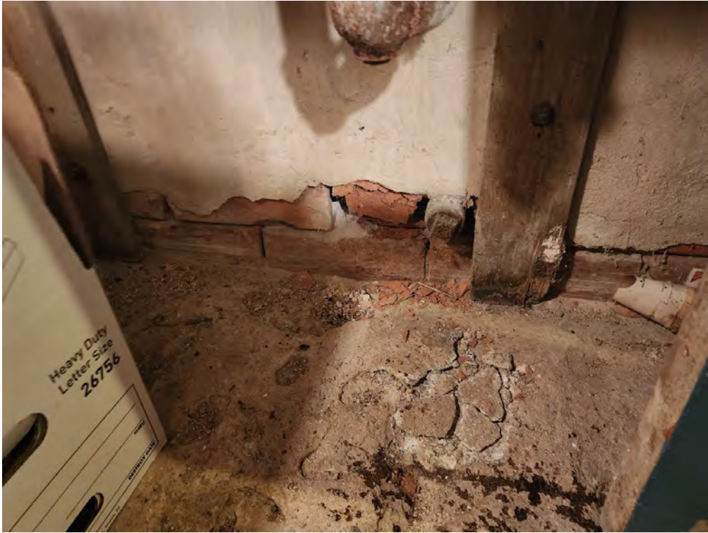
Cracks under darkroom sink
