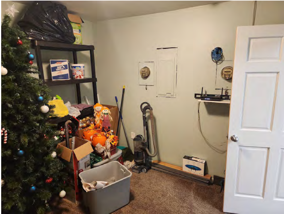
Electrical in storage
