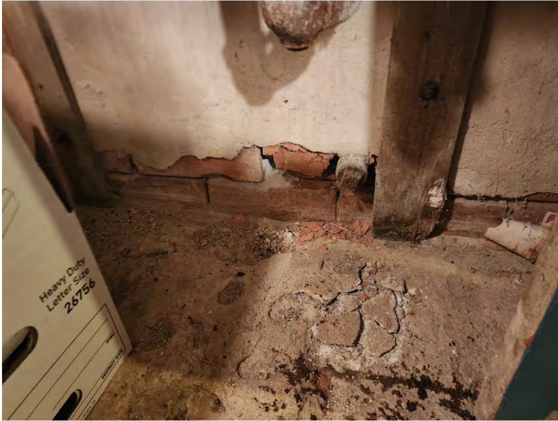
Cracks under darkroom sink
