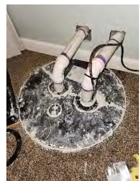
Photo 4: Airtight sump with sampler
