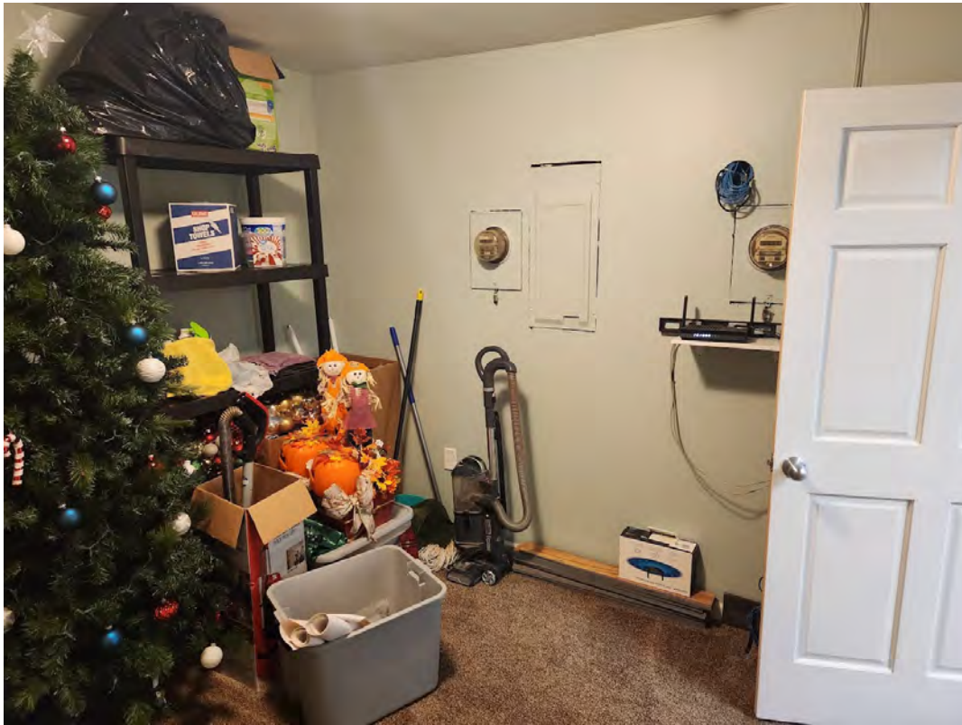
Electrical in storage
