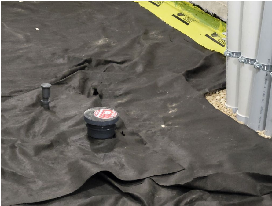
Photo 7: VP-1 installed in electrical room (to the left of the floor drain) prior to completion of the vapor barrier (10/5/2023; 17:49).
