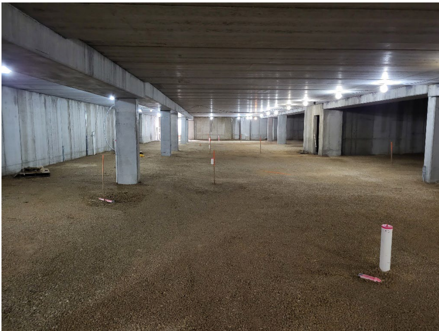
Photo 4: Gravel drainage layer prior to placement of vapor barrier, looking toward the southwest corner of the building (9/29/2023; 12:25).
