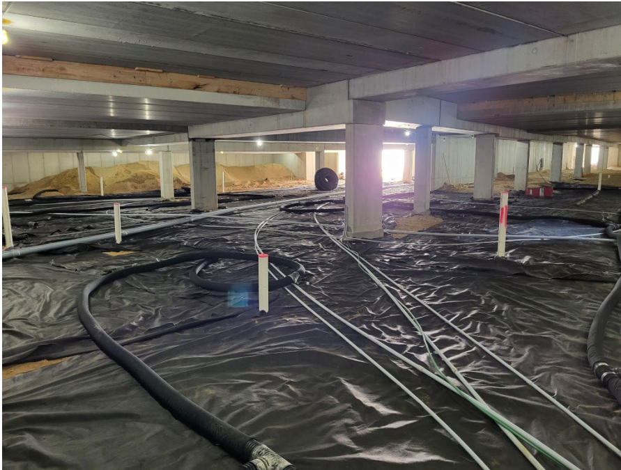
Photo 3: Lower level floor/parking area with a partially completed drain/vent piping looking southeast toward parking ramp entrance (9/18/2023; 14:19).
