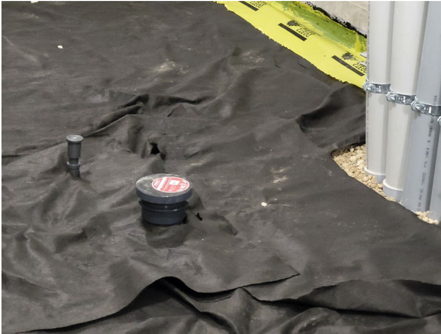
Photo 7: VP-1 installed in electrical room (to the left of the floor drain) prior to completion of the vapor barrier (10/5/2023; 17:49).
