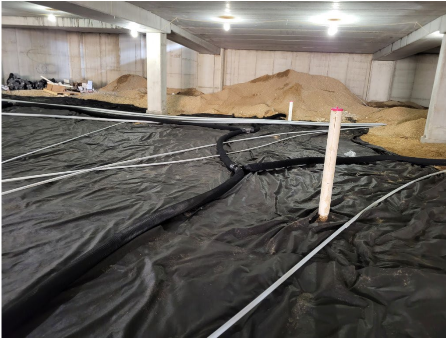
Photo 1: Lower level floor with drainage/vapor piping (black), electrical conduit (gray), and rough plumbing (white) (9/18/2023; 14:15).
