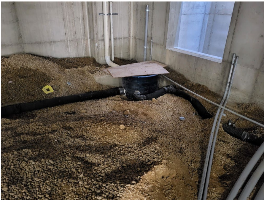
Photo 2: Sump at the northeast corner of the lower level with drain/vent pipes connected and opening for ventilation fan visible to the right of the sump (9/18/2023; 14:16).
