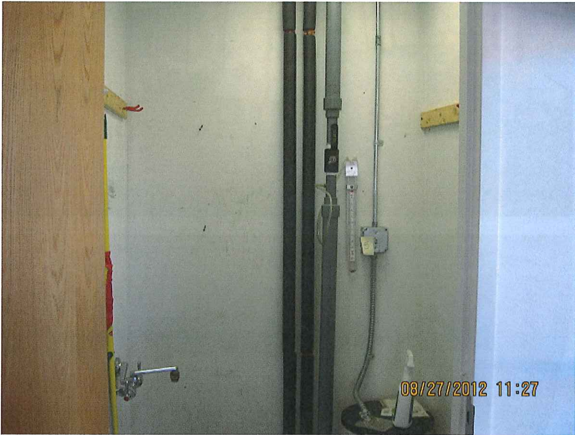
Vent pipe ball-valve in re-opened position; empty manometer to right of valve.
