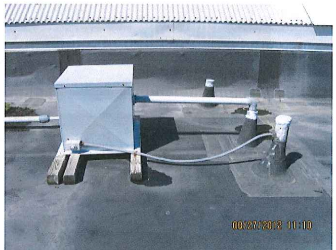
Depressurization blower in galvanized box; vent pipe in on right, out on left.
